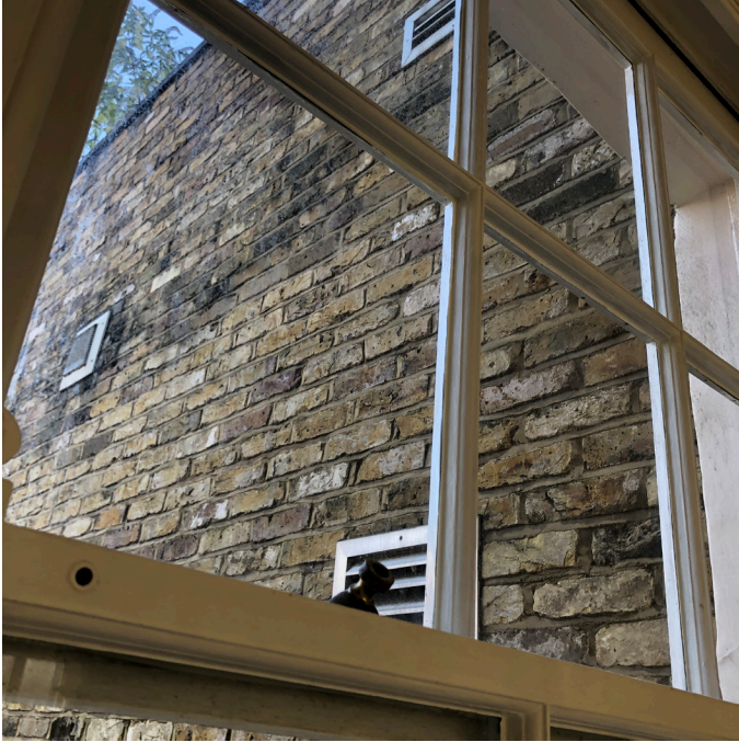
ventilation grilles scattered across N-E elevation of closet wing N°26 Lower Belgrave St
