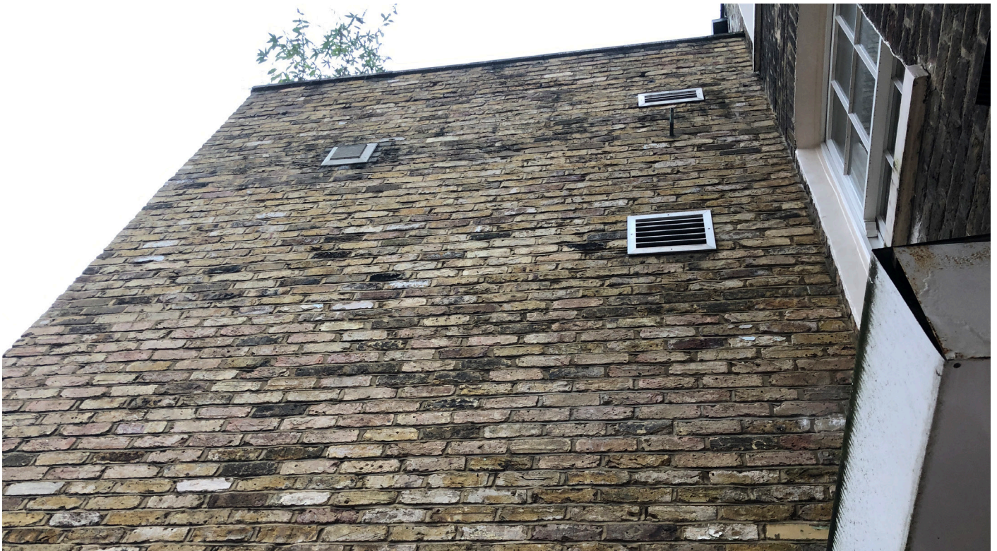
N-E elevation of closet wing seen from ground floor Patio N°26 Lower Belgrave St
