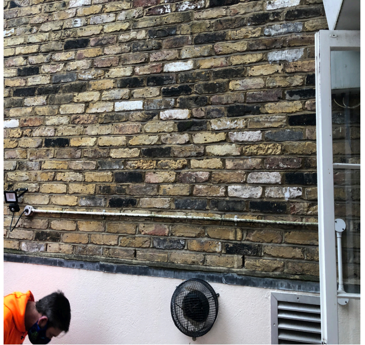
boiler extract and ventilation grilles within rear Patio N°26 Lower Belgrave St
