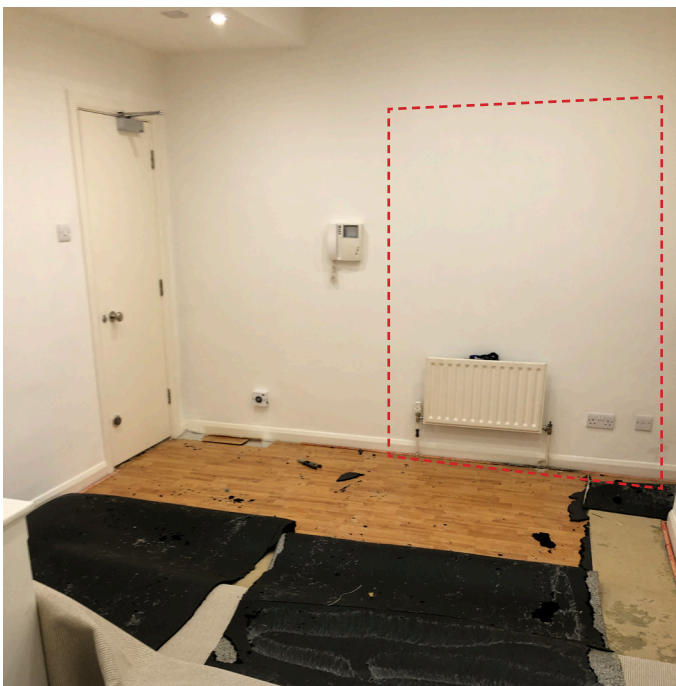
existing wall between future Playroom and TV Den, with new opening outlined in red
