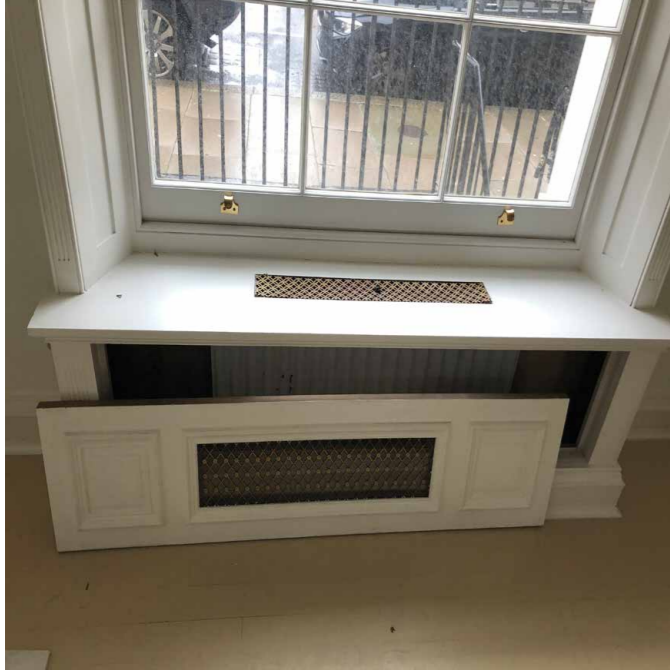
existing radiator and case
