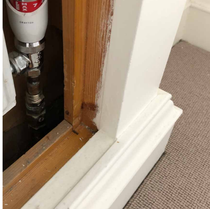
existing radiator and case (RT.01, RT.02)
