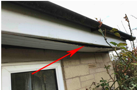
Photo 3: Red arrow points to opening beneath soffit. Eastern gable wall.
