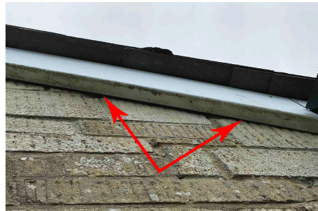
Photo 4: Red arrows point to gaps beneath plastic fascia. Western gable wall.
