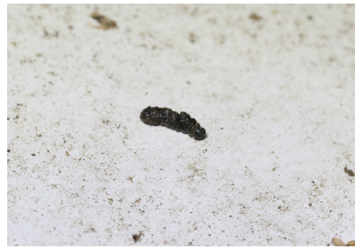
Photo 8: Bat dropping discovered in main loft element.
