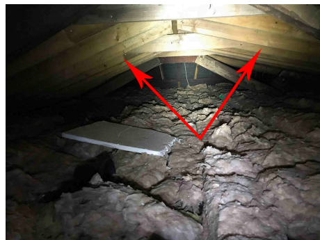
Photo 6: Red arrows point to exposed timber joists and purlins of roof structure within loft void.
