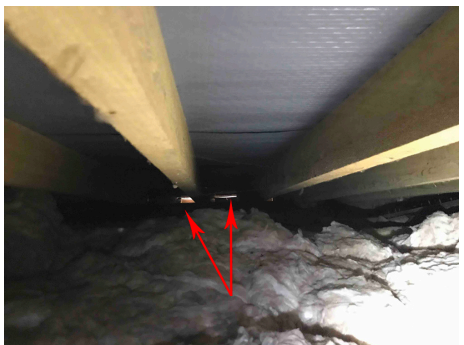
Photo 5: Red arrows point to daylight visible within the loft void.
