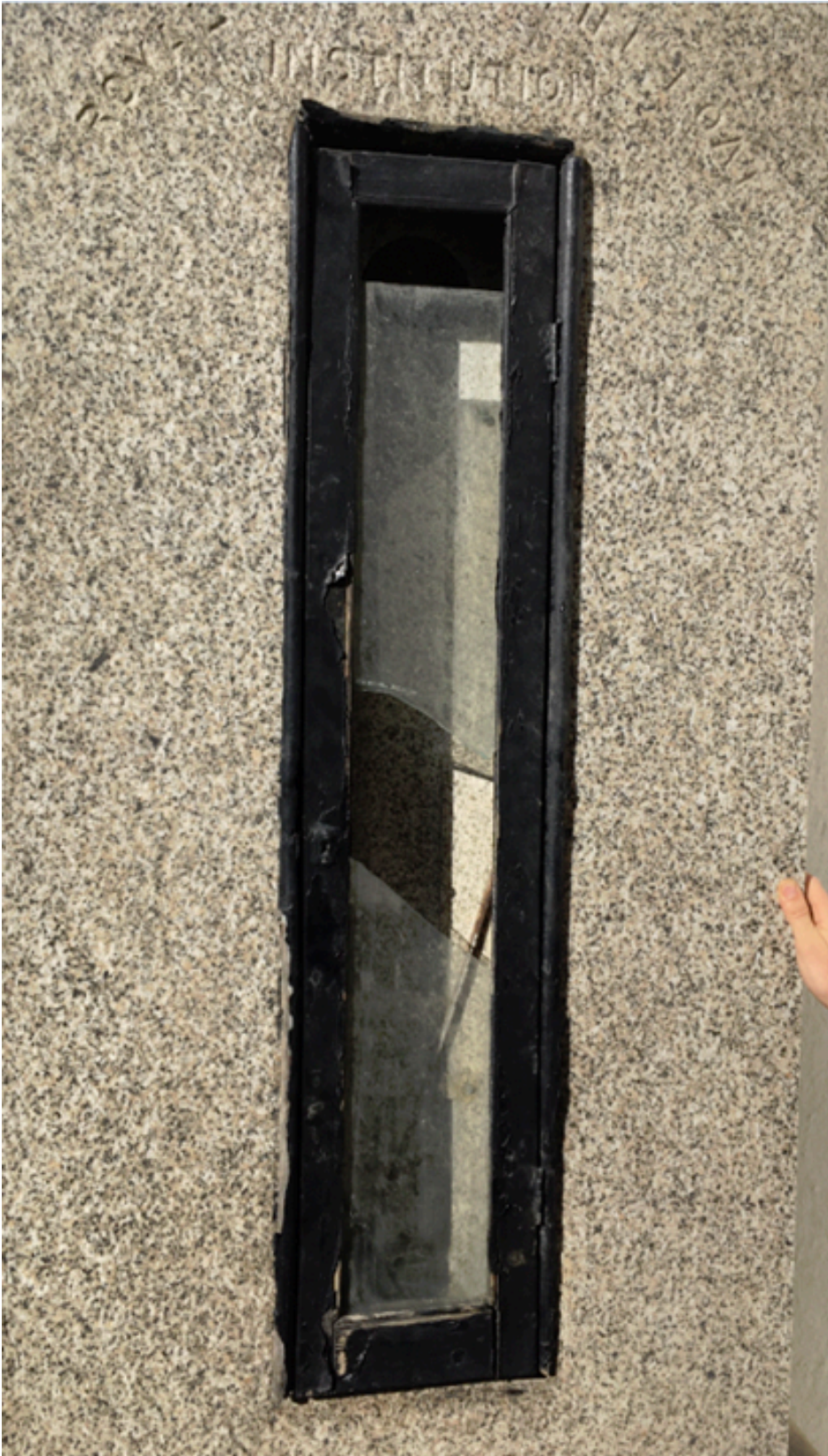
The existing housing door in badly damaged wood and broken glass.
