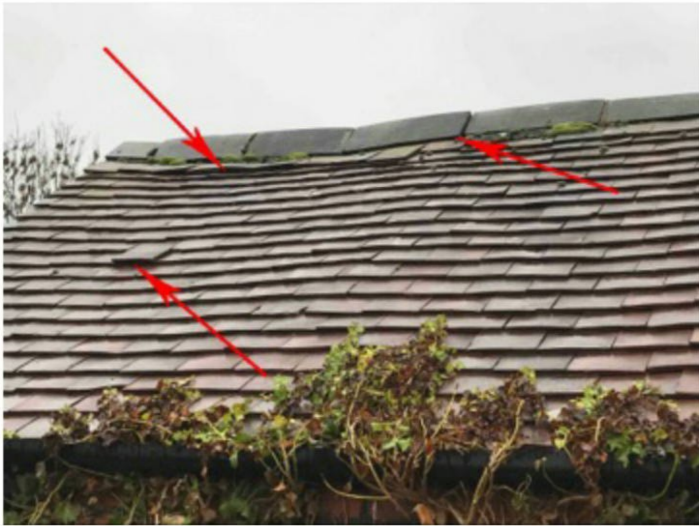
Photo 7: Red arrows point to gaps beneath roof tiles and ridge tiles. B2.
