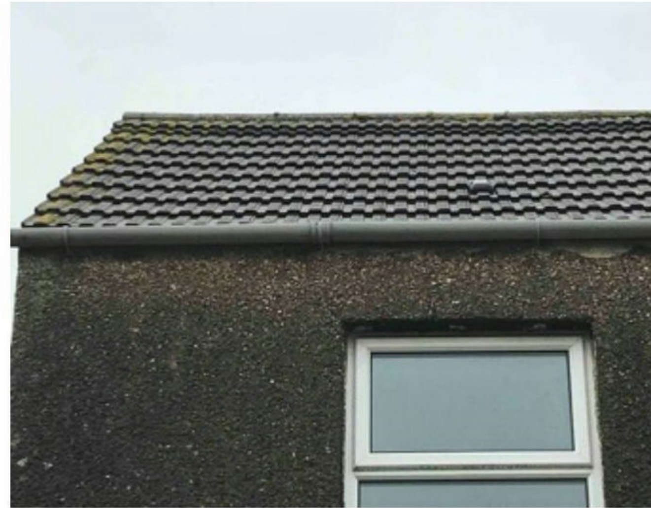
Photo 2: External roof of B1, which was in good condition without any obvious slipped or raised roof tiles.
