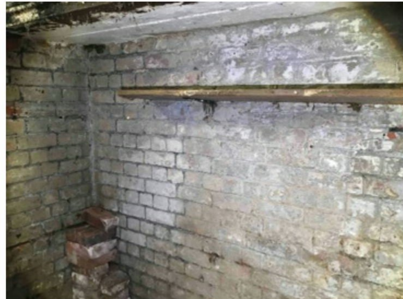
Photo 10: Internal brick walls of basement were in good condition without cracking. B2.
