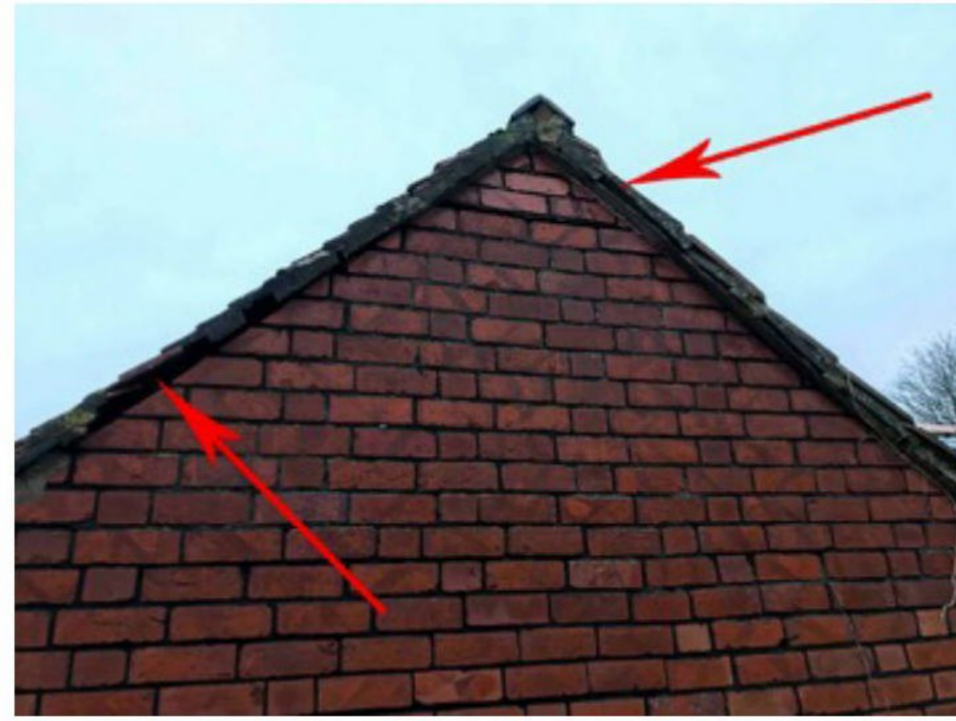
Photo 8: Red arrows point to gaps caused by failed mortar at southern gable wall. B2.
