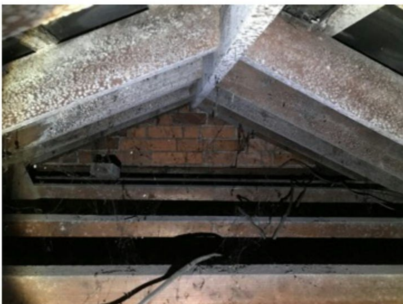
Photo 5: Internal view of small and shallow loft space above single-storey element of B1.
