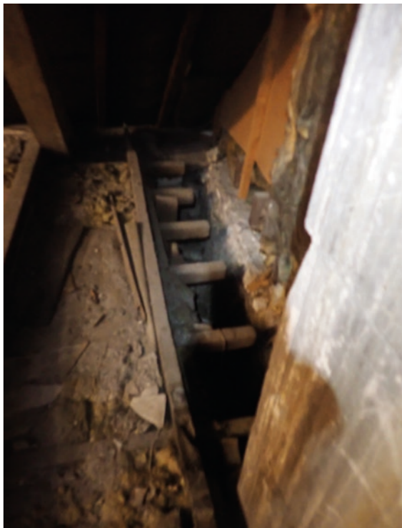
View 73: View down over built in cupboards in front bedroom over shop 1
