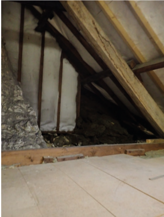
View 66: Attic looking north showing existing chimney, party wall and rear roof slope
