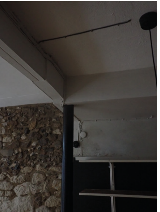
View 50: Internal view of Shop 1 - steel column supporting first floor chimney hearth
