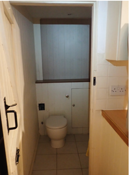
View 55: Existing low ceiling over WC accessed off the kitchen.
