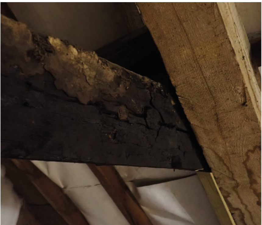
View 68: Existing charred timbers
