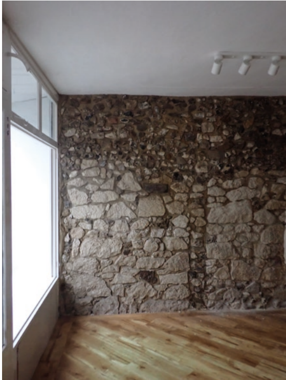
View 46: Internal view of Shop 1 showing exposed stonework and internal window framework
