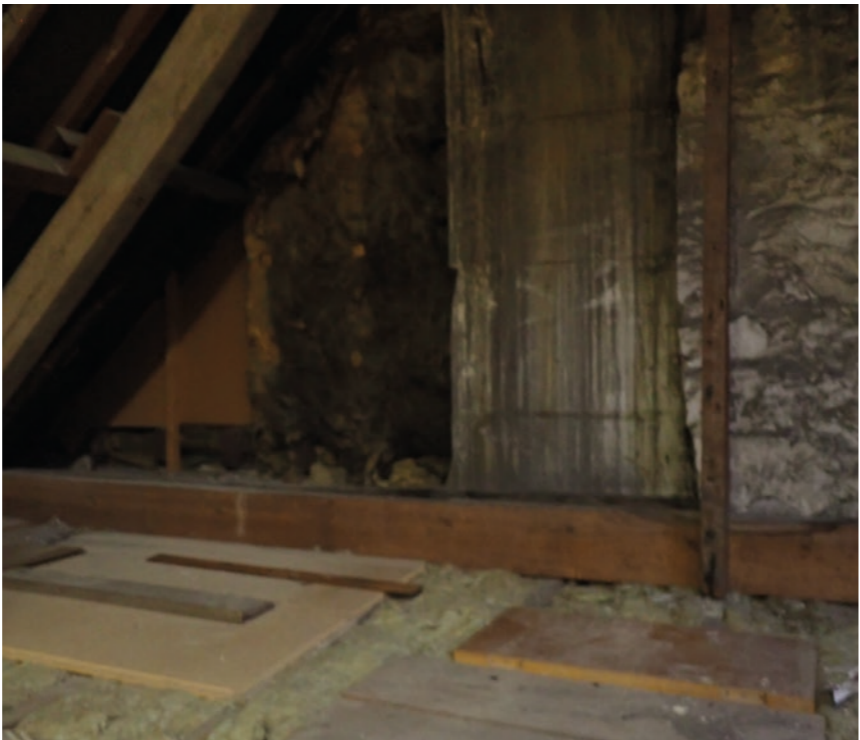
View 67: Attic looking north showing existing chimney, party wall and front roof slope
