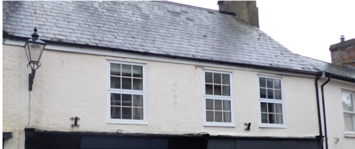
View 5: The existing upvc mock georgian top hung windows, and Victorian Gas lamp styled street light
