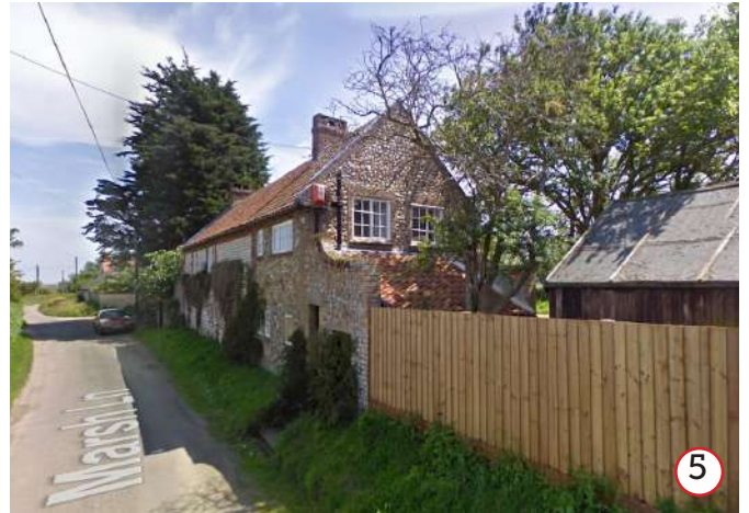
View East towards Denning's Western gable, noting modern timber fence and dilapidated timber shed to rear, which makes no positive contribution to streetscene. Note also grassed bank to highway, which is to be retained.
