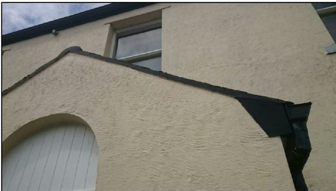
Photograph 20 showing the roof edge of the entrance on the eastern side of the building
