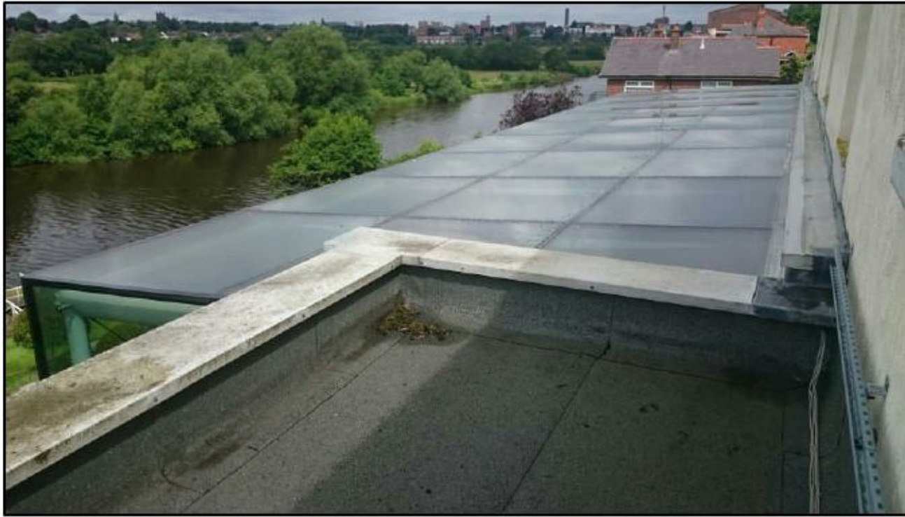
Photograph 13 showing the roof of the glass extension to the rear of the property
