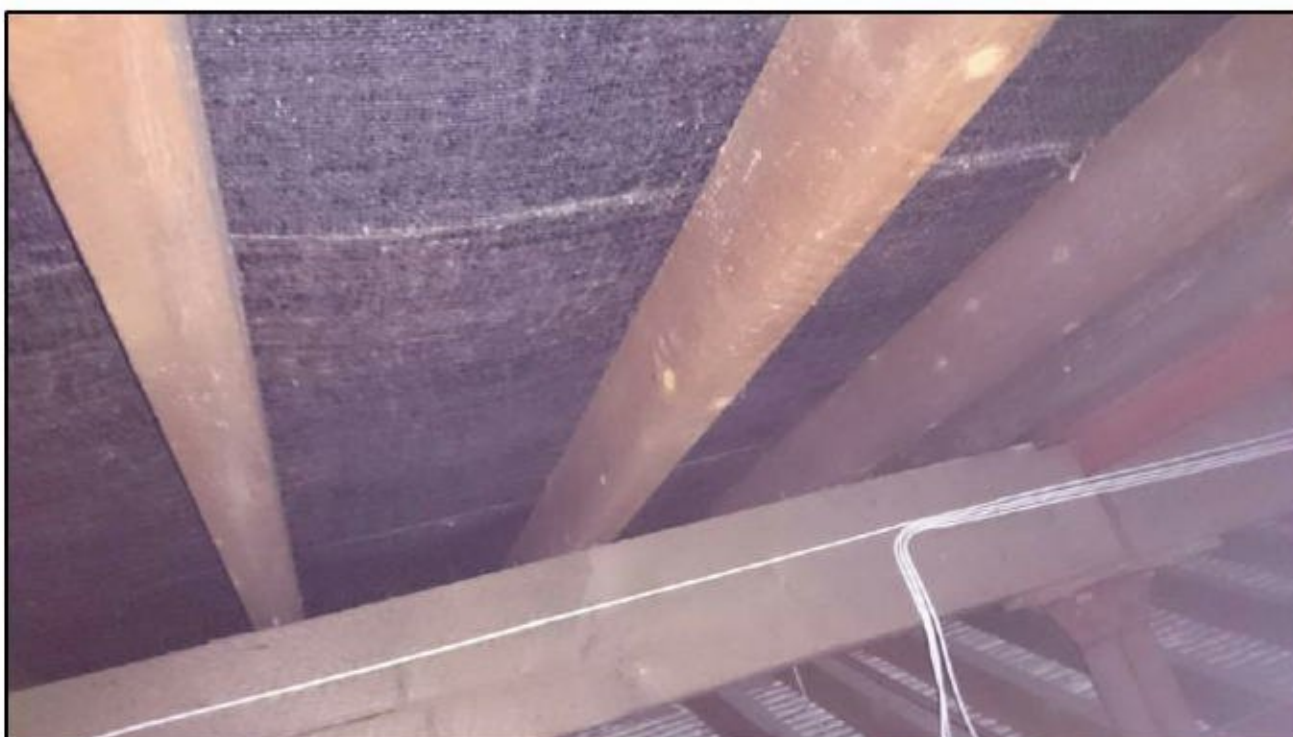
Photograph 27 showing a section of roof felt
