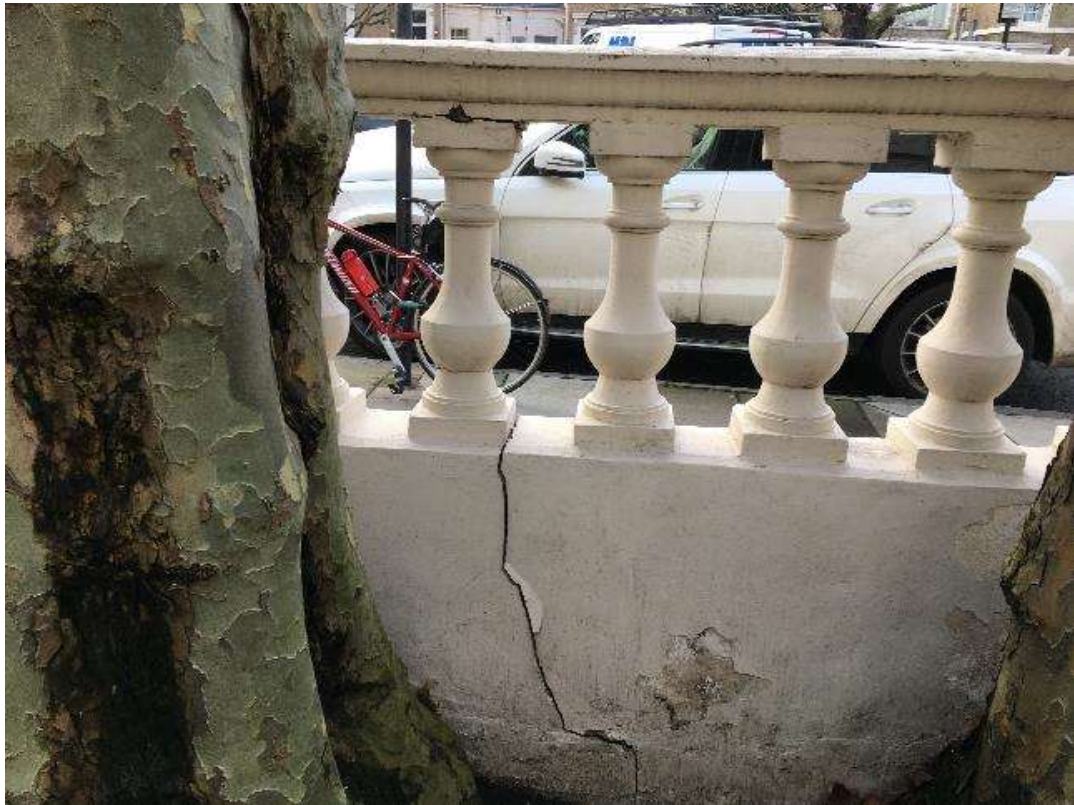
Photo 8: Detail of cracked middle section of wall.
