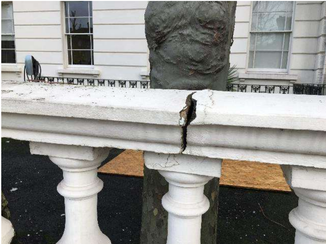
Photo 10: Detail of cracked top rail to middle section of wall.
