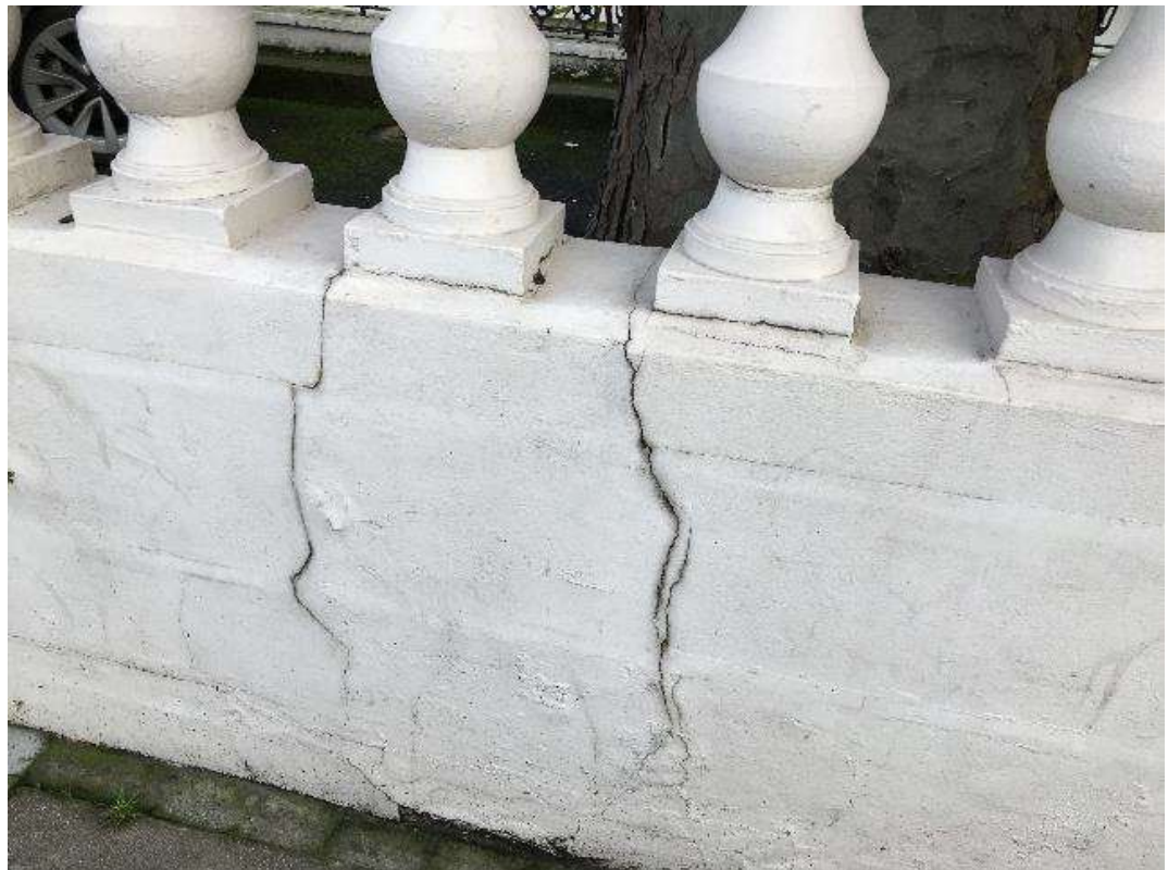
Photo 9: Detail of cracked middle section of wall.
