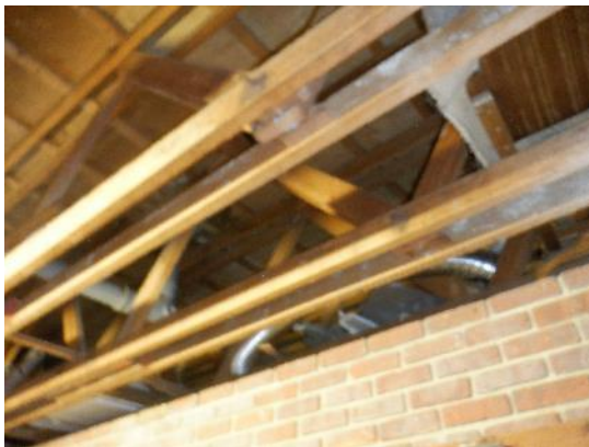
37. Open void section above rooms to the western side of the garage.
