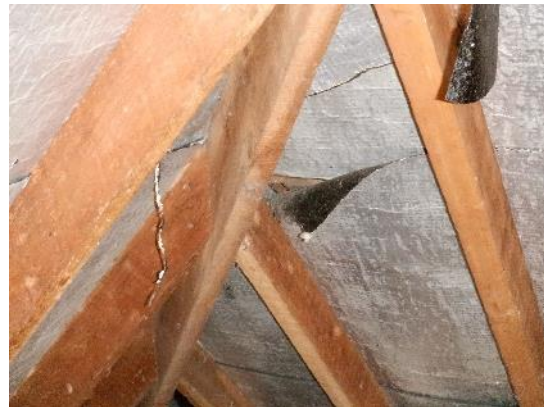
22. Tear in foil covered bitumen felt roof lining.
