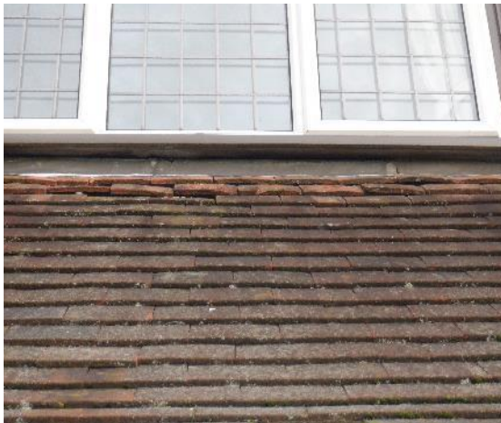
11. Lifted roof tiles below rear dormer window.
