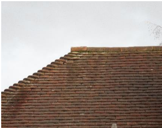
9. Gaps between roof tiles near corner of ridge and hipped tiles.
