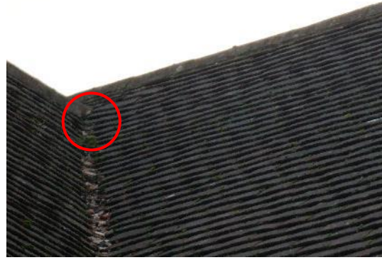
8. Lifted roof tile below ridge tiles of pitched roof.
