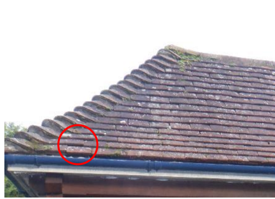
18. Lifted roof tile on western elevation of the hipped edge of the garage roof.
