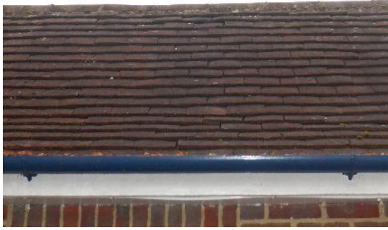
19. Occasional lifted roof tiles on southern elevation of the garage roof.
