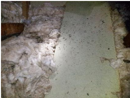
21. Fibreglass insulation on the floor of the void with occasional boarding along western side of the void.
