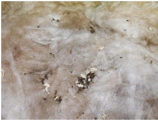
33. Scattered bat droppings on fibreglass across the southern section of the void.
