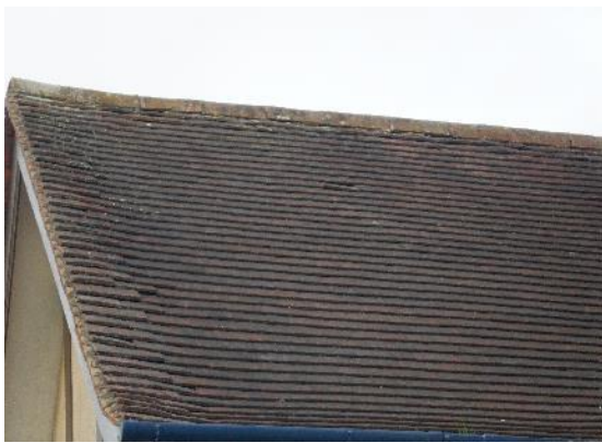
15. Lifted roof tiles below ridge tiles; gaps where verge tiles have moved apart.
