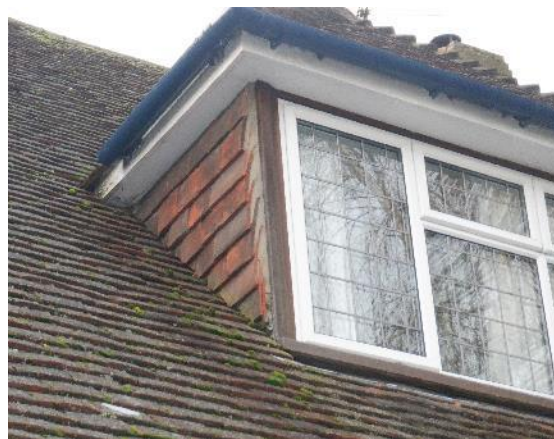
6. Slightly lifted hanging tiles on southern dormer window.
