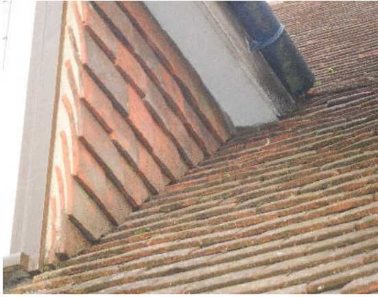
13. Occasional lifted hanging tiles around dormer window on rear elevation.
