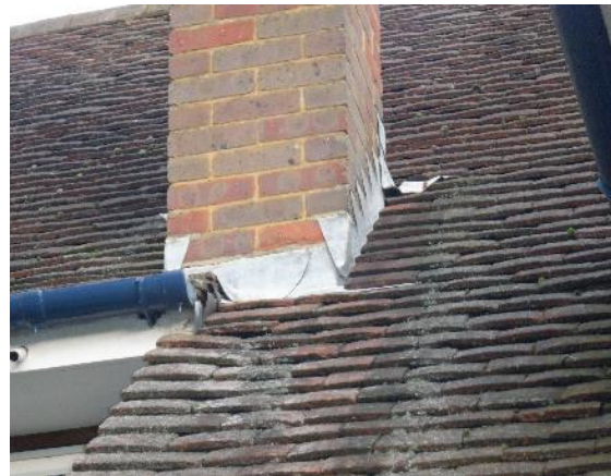
10. Lifted roof tiles and lifted lead flashing around the base of the chimney.
