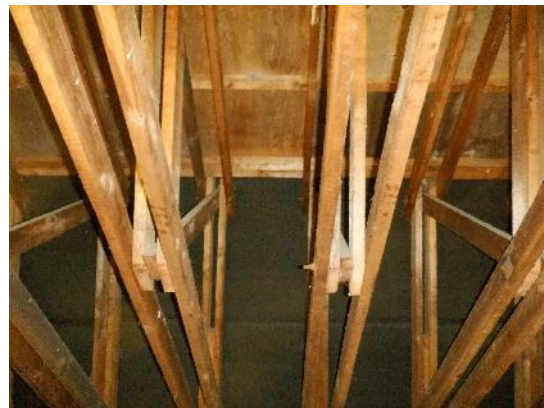
38. Roof tiles lined with tight bitumen felt and wooden boarding lining the flat section of the mansard roof.
