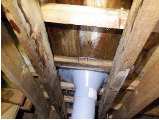
39. The westernmost drainage pipe on the flat roof, with water damage on the boarding around the top.
