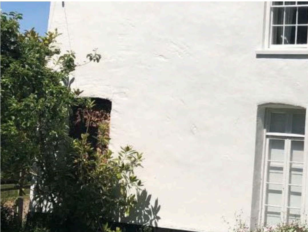
2.2. View of exterior wall to sitting room facing north - original door opening can be seen on left (infilled with stone)1a. Interior view of sitting
