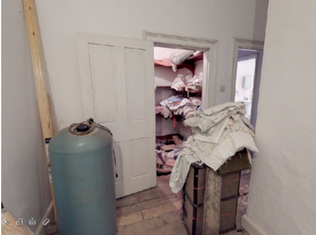
2.8. Part of partition walls to be removed. floor boards in this area are narrower and door frames inconsistent.
