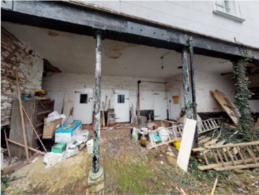
2.7 Existing wrought iron columns within central service yard - glazed screen to be inserted behind.
