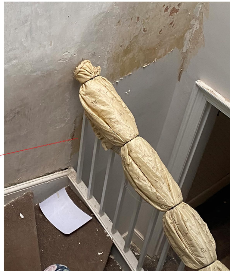
2. Ground floor handrail abuts the wall with a less elegant detail.
