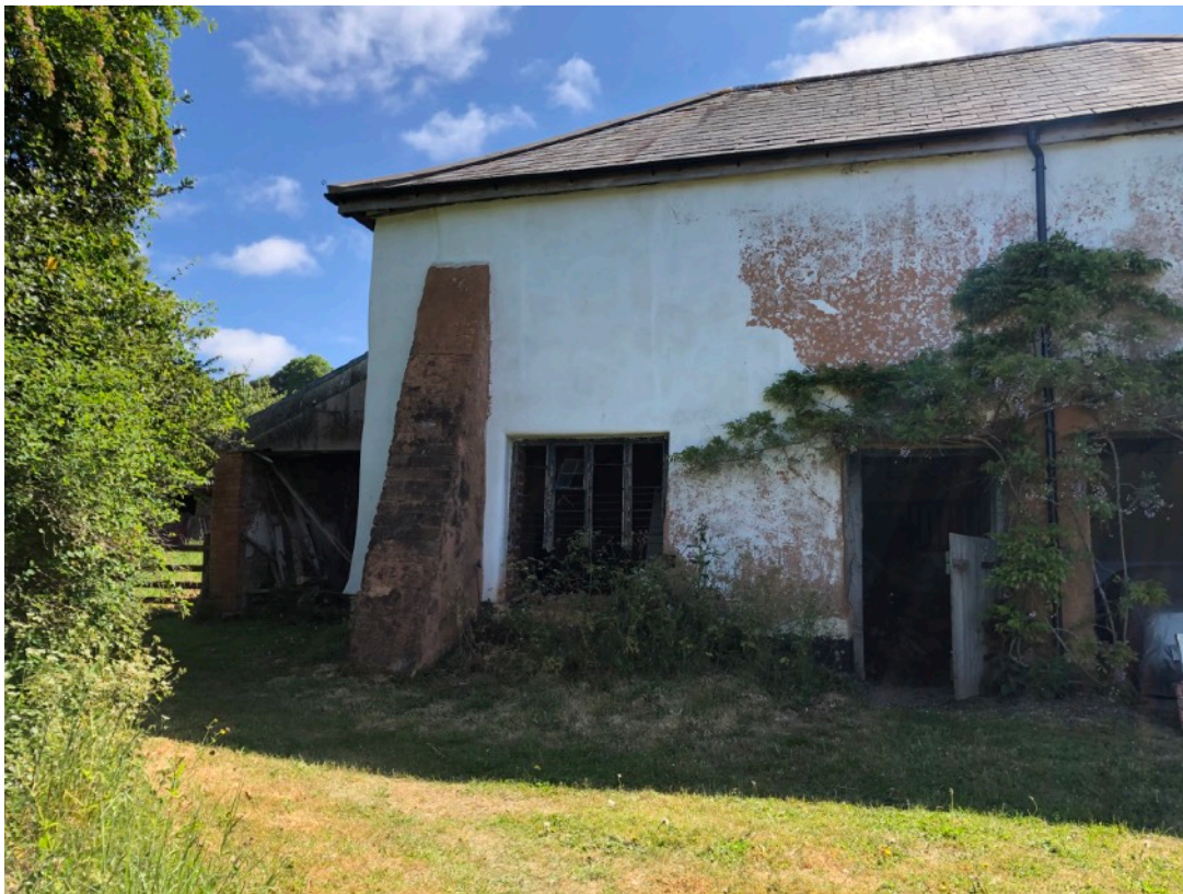
1.12 View of 2-storey barn - lines of previous opening can be seen above existing window opening.
