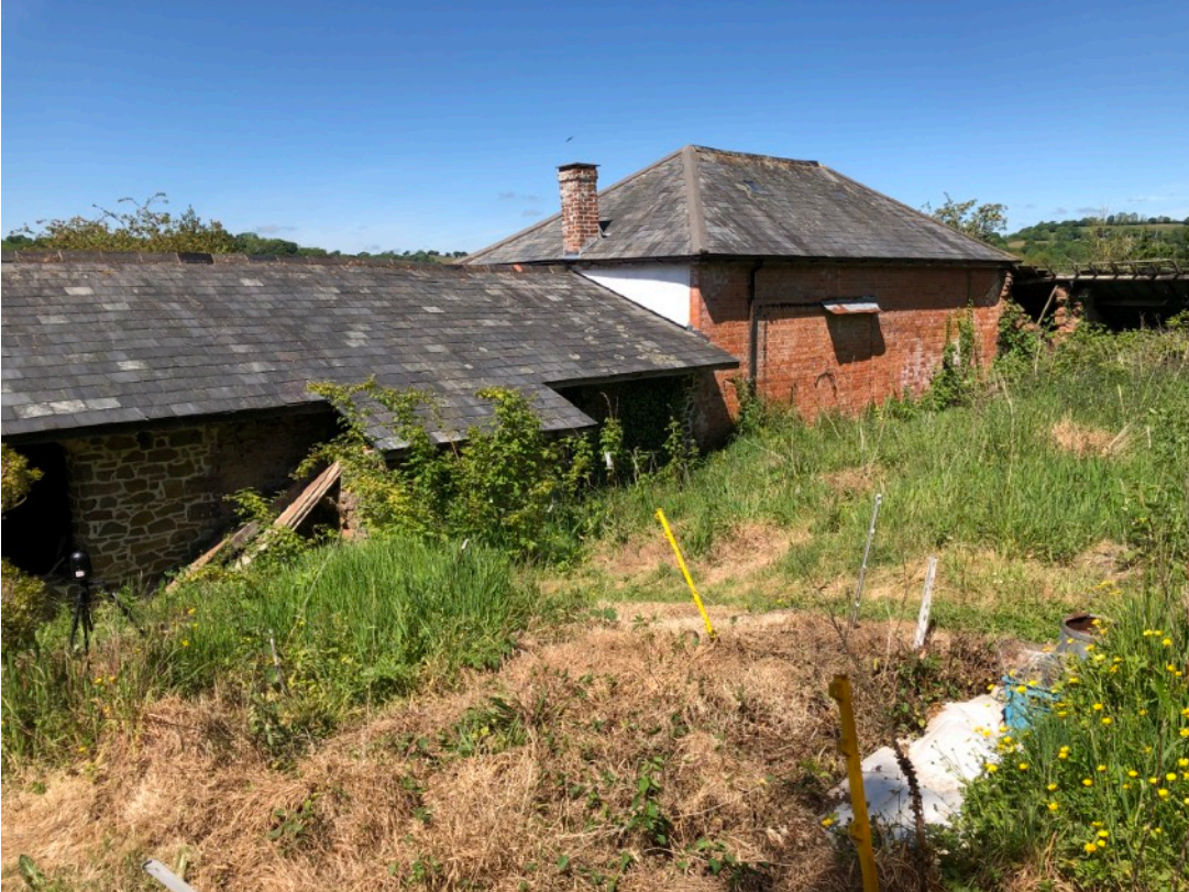
1.16 Barns from rear looking north-west - derelict stable to right.
