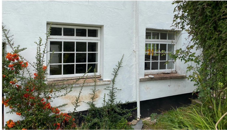
WG05 & WG06 Existing photo Windows are C20 replacements with top opening casements.
