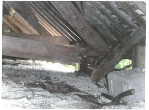
Broken A frame - barn
