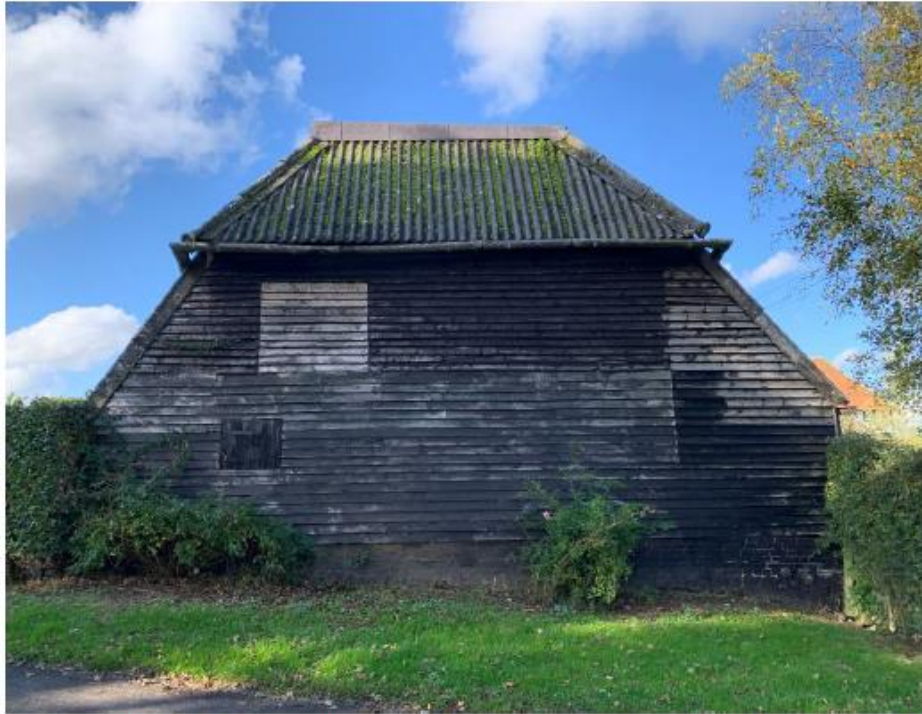
Photo of the southern elevation of the barn showing the patchwork of new and old boards.
