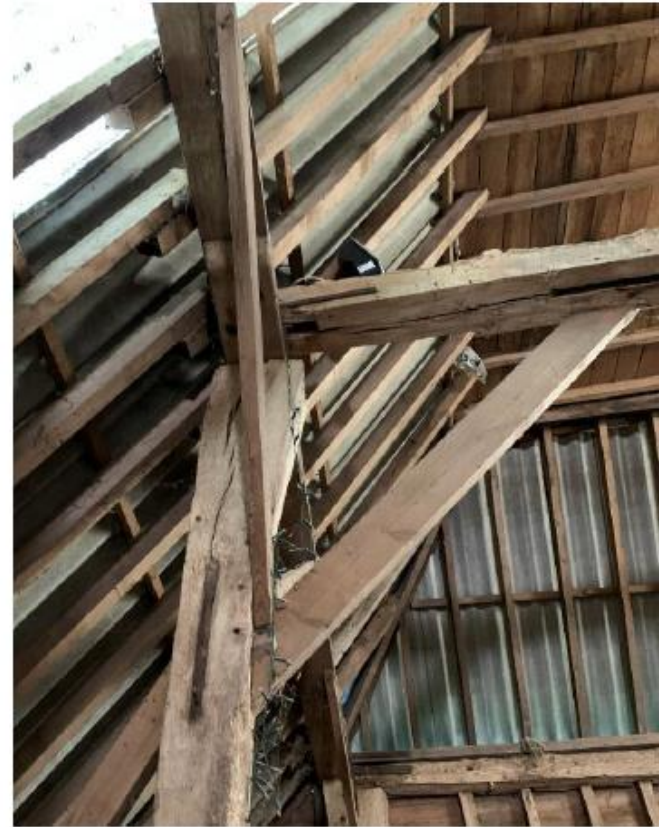
Photo of frame 5 on the eastern post, showing the typical 1960's sawn timbers.
