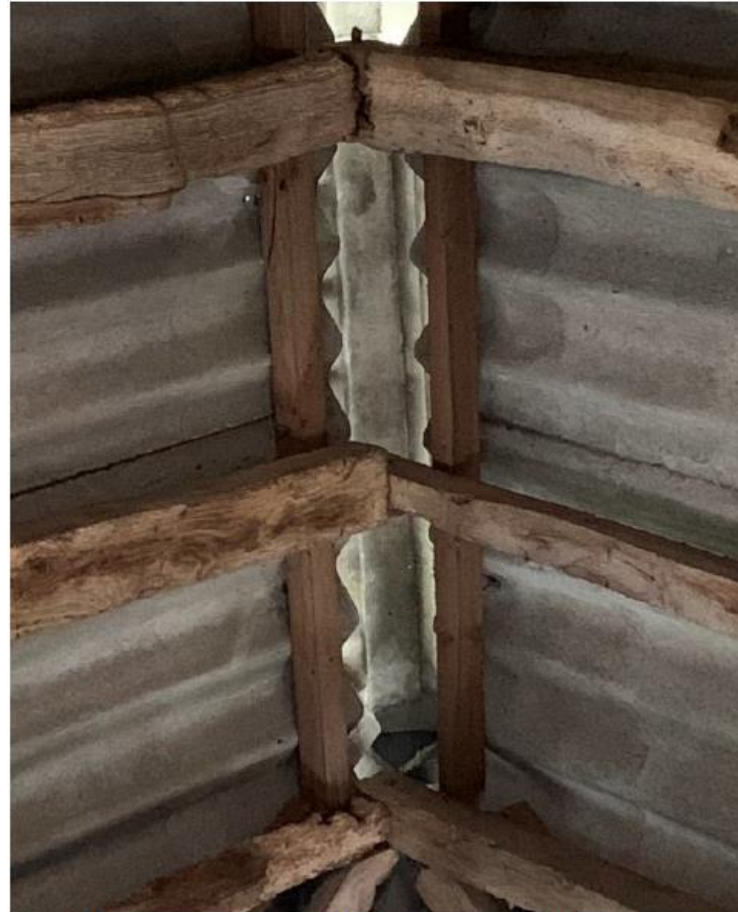
Photo of the timber joint detail in the apex of the roof of the cart opening.
