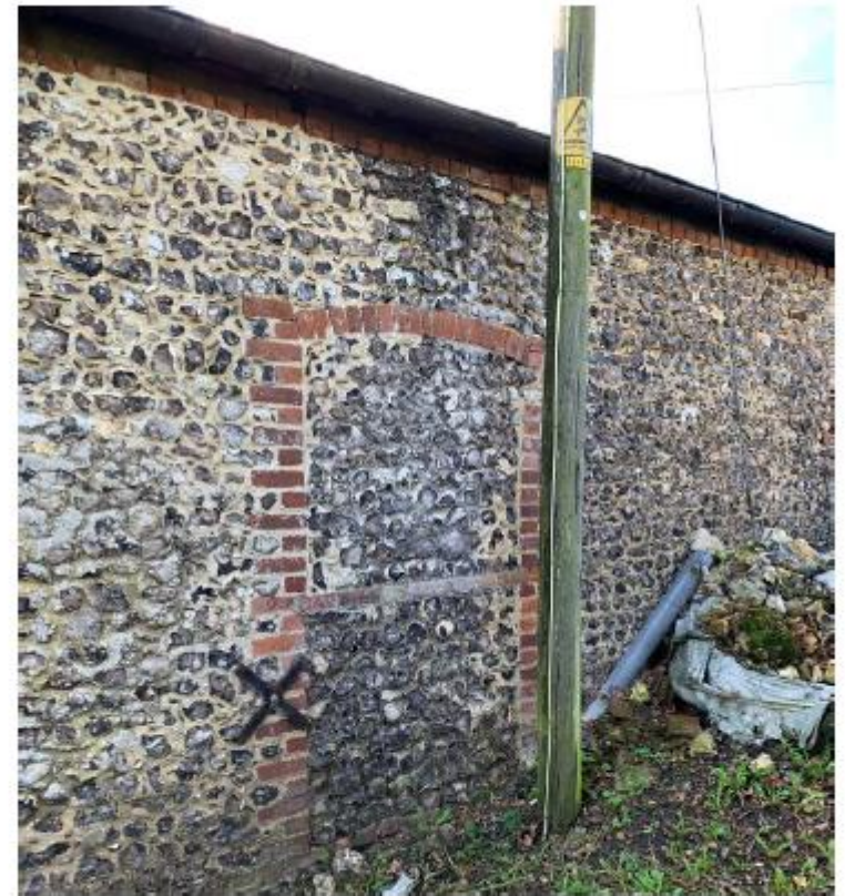
Photo of the eastern wall of the single story building, showing the historic opening and the steel wall restraint.
