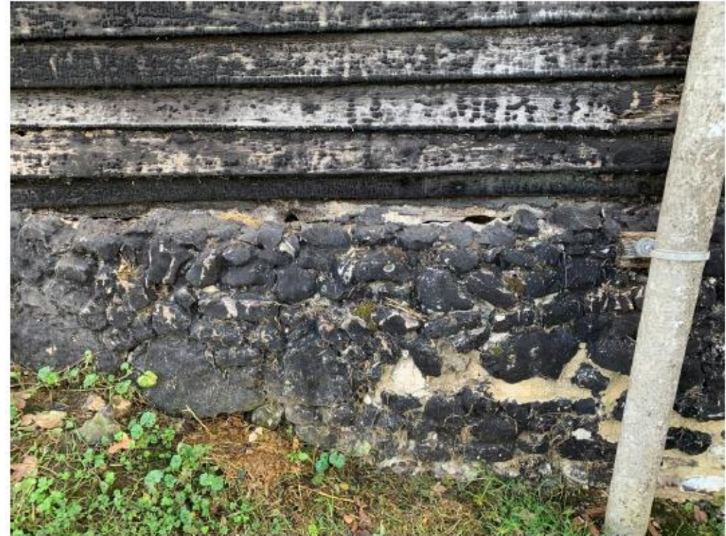
Photo of the north-eastern length of the base wall, this is typical of the poor condition of the wall.
