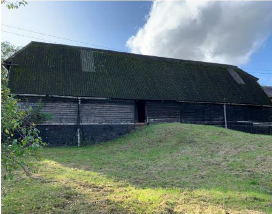
Photo of the eastern elevation showing the raised ground for access into the barn.
