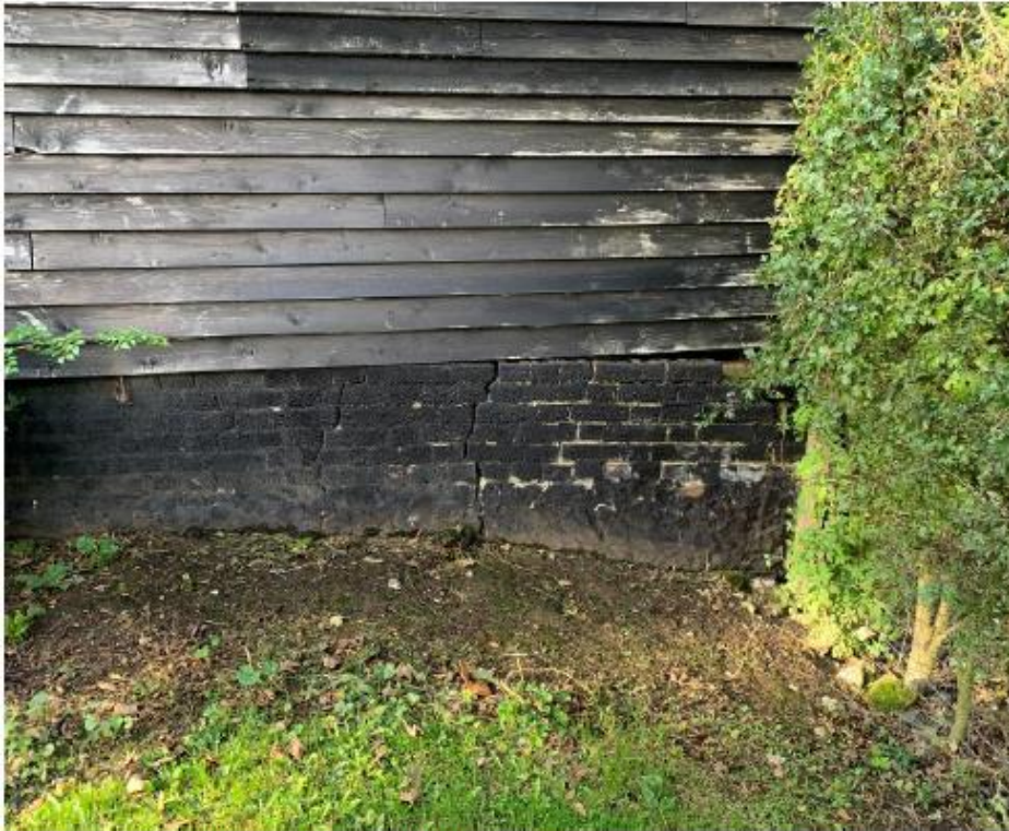
Photo of the south-east base wall where there are signs of movement.
