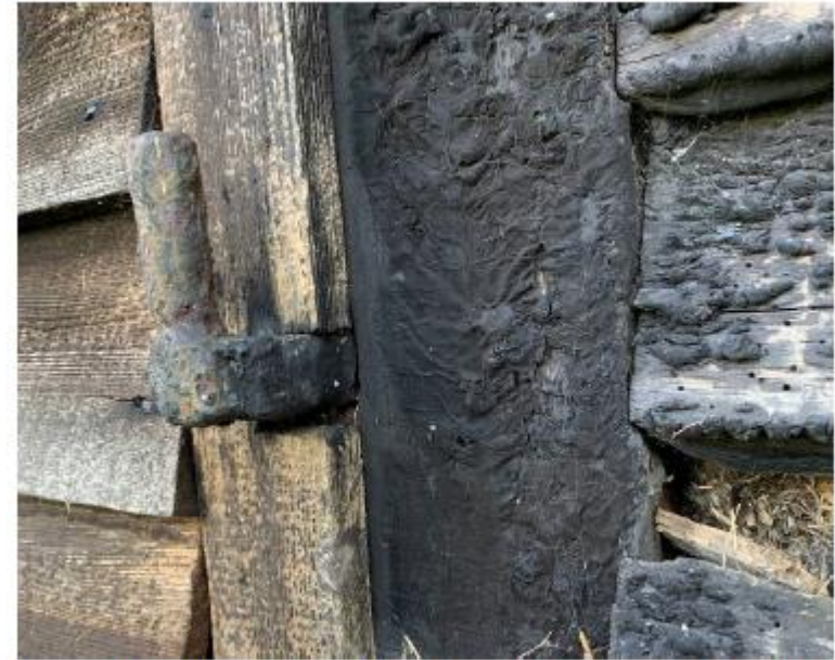
Photo of the remaining pintle on the northern side of the opening.
