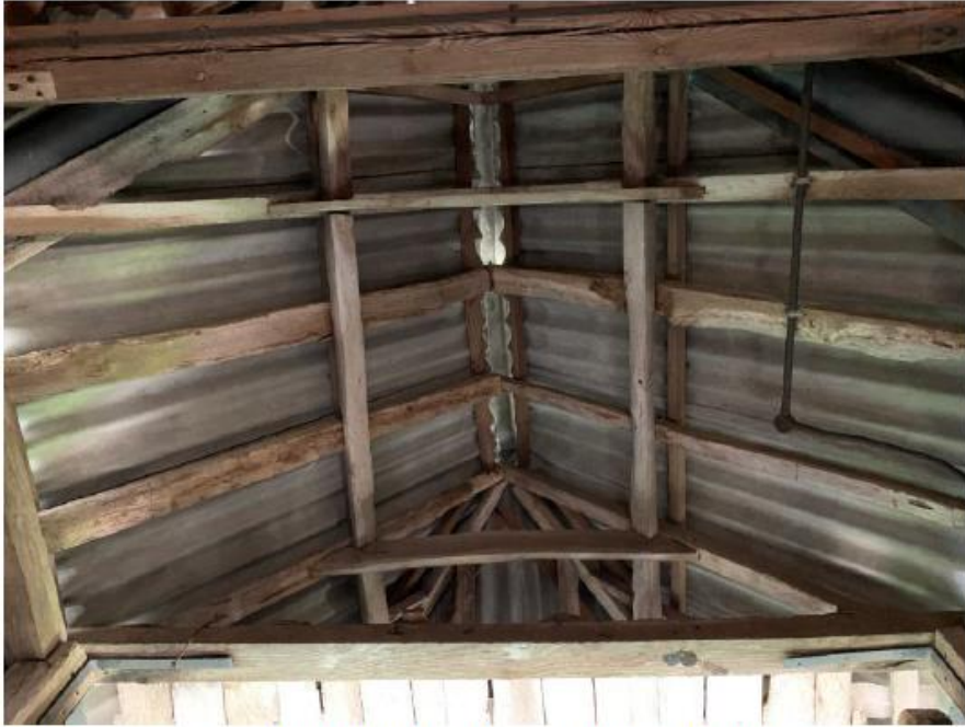
Photo of cart entrance roof showing the rafter and purlins with tie beams.
