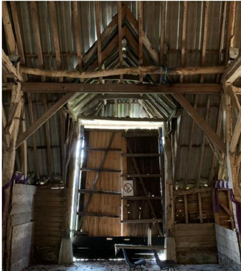
Internal photo of the timber door to the cart entrance on the eastern elevation.
