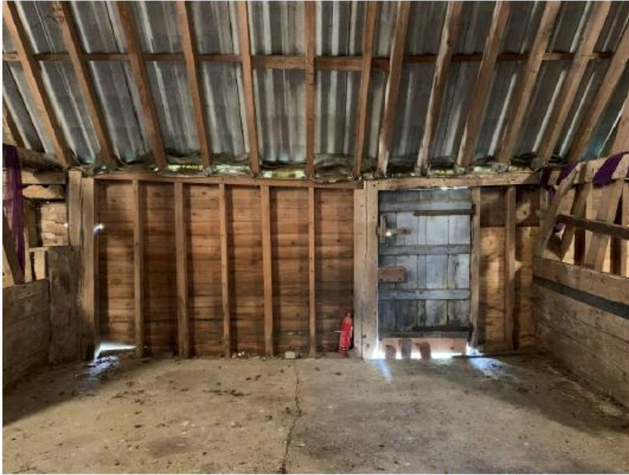
Internal photo of the in-filled opening on the eastern side of the building.
