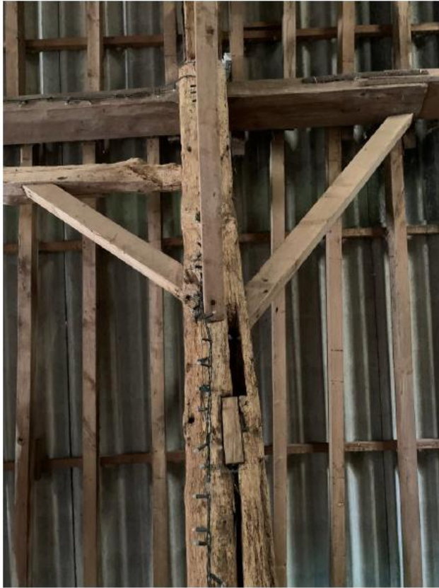
Photo of east post and nailed and sawn timber braces of frame 4.
