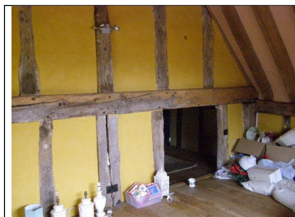
Existing low level opening between Bedrooms 1 & 2 – This opening is to be maintained.
