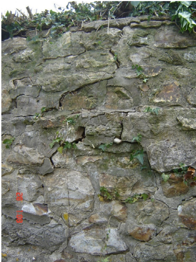
Cracks in wall prior to collapse.
