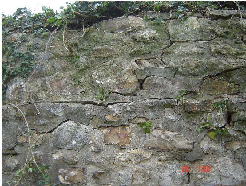
Cracks in wall prior to collapse.
