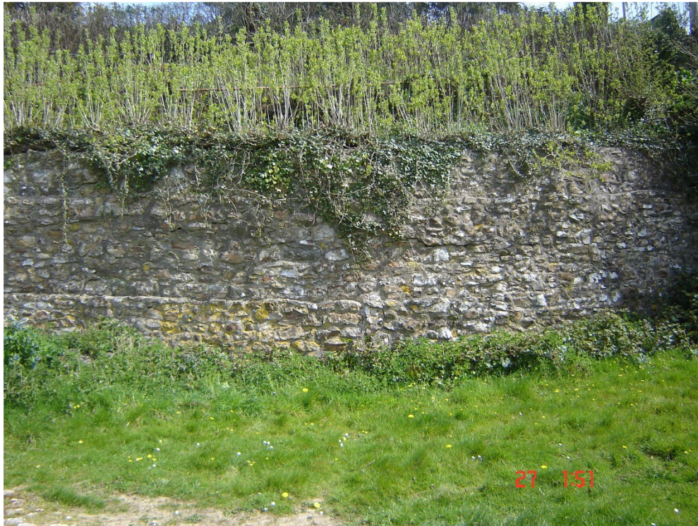
Existing masonry wall from farmyard prior to collapse.
