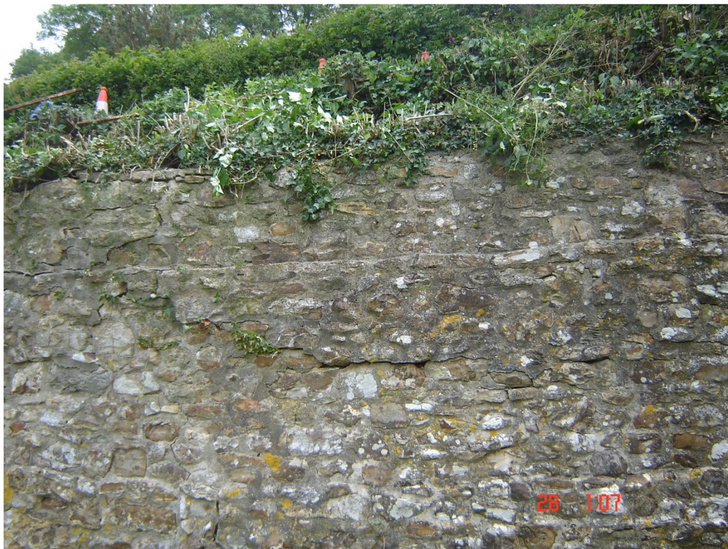
Cracks in wall prior to collapse
