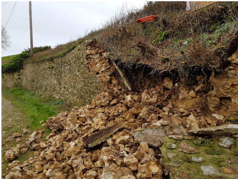
Collapsed wall – January 2021
