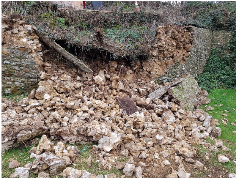
Collapsed wall – January 2021
