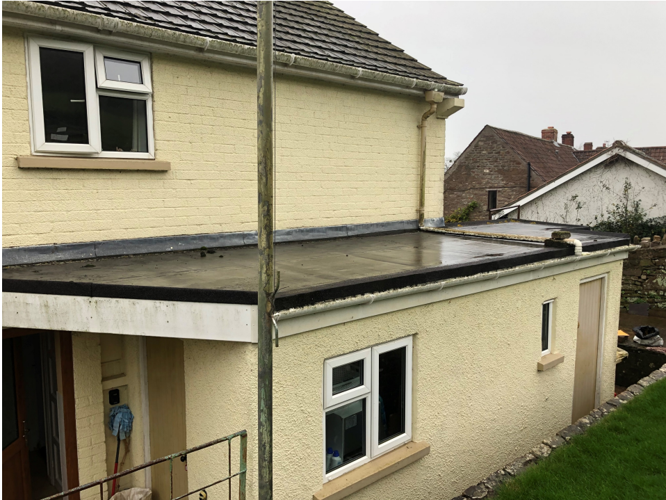
Poorly built single storey extension to rear
