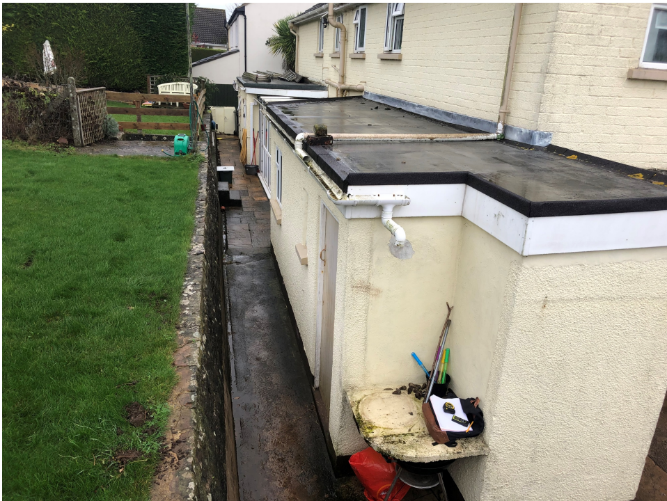
Narrow passageway between garden retaining wall and rear wall of single storey structure
