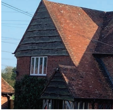
Generous sized timber planking gives a feel of quality, bespoke and traditional build.
