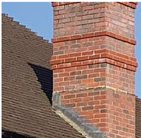
Traditional Brick Chimneys for wood burning stoves?
