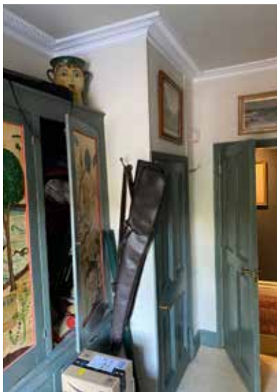
The south-eastern corner of the present cloakroom; the corner enclosure and all the joinery and cornicing is modern
