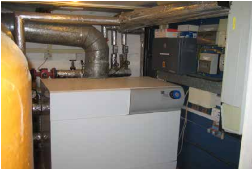
The present boiler room in the basement
