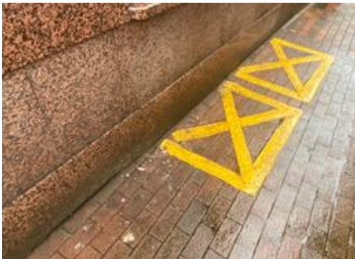
Image 2: Fouling at the side of the branch near the ATM
