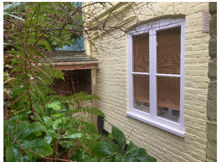
Figure 3 Close up of the rear wall and the potting store that will be replaced by the heat pump
