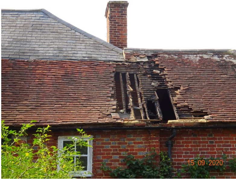
Damaged roof over north wing.
