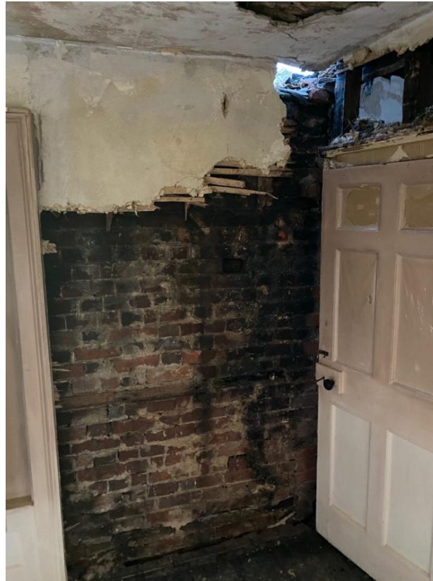
View of fire damaged structure in bedroom 5
