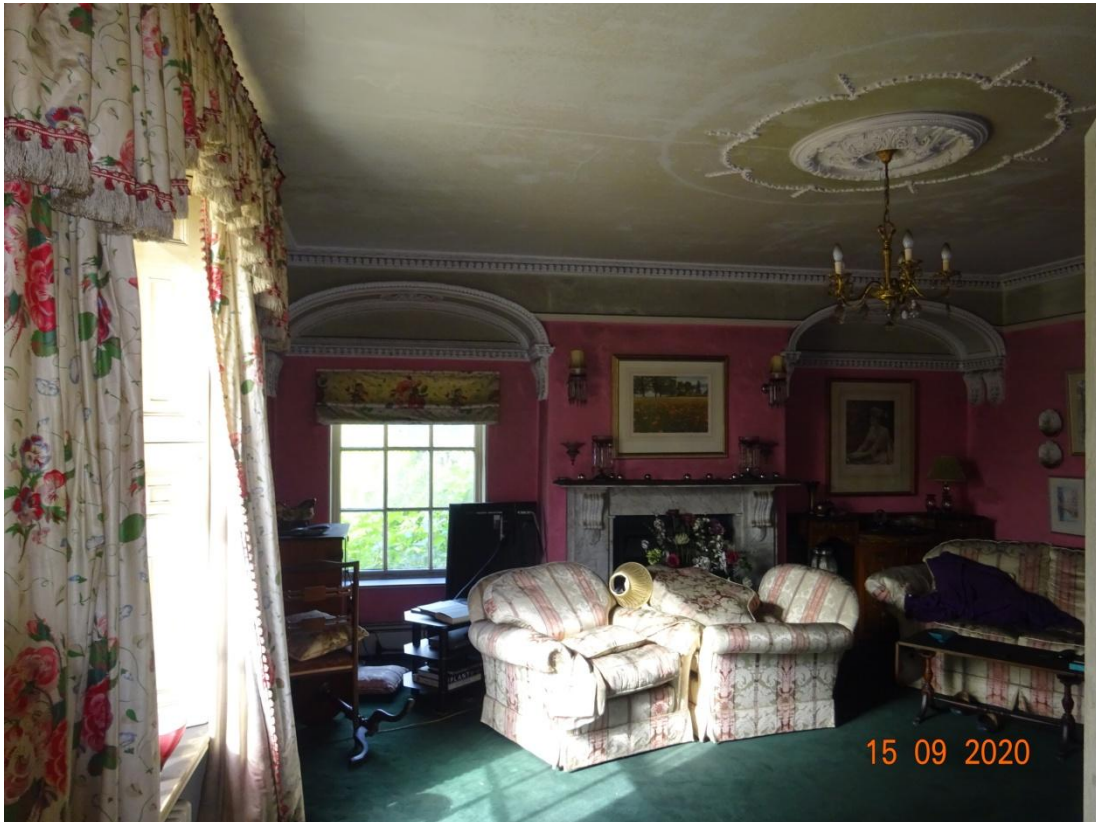
Living room after fire
