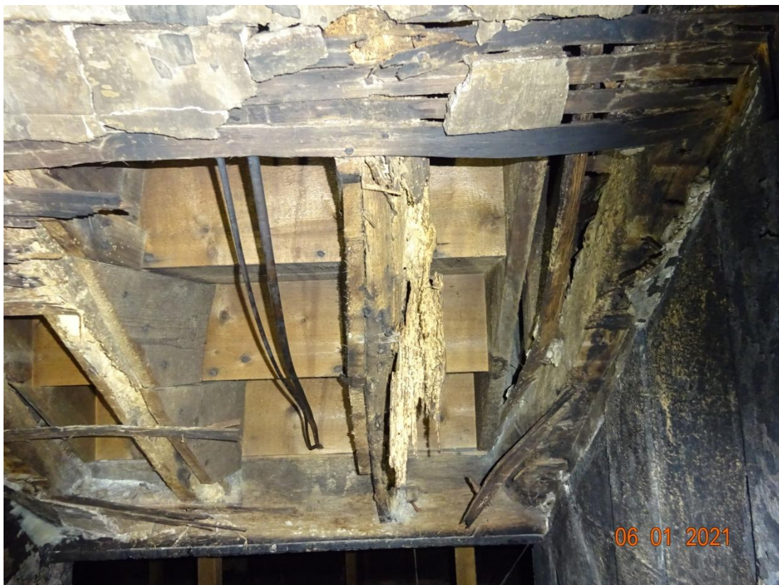
Detail of deteriorated and infected timber stairs from bedroom 5 to the hall on the first floor
