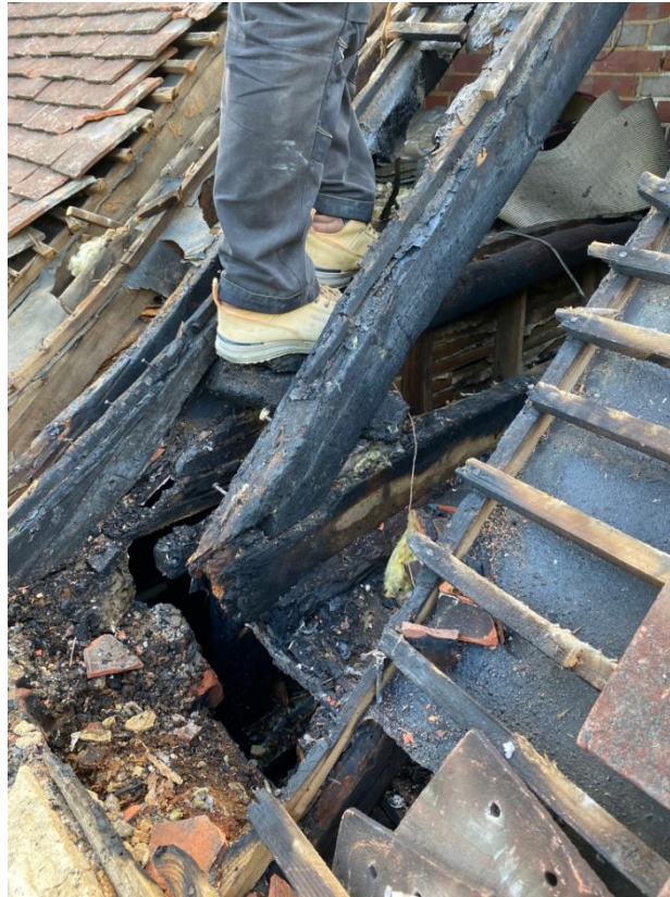
Detail of damaged roof
