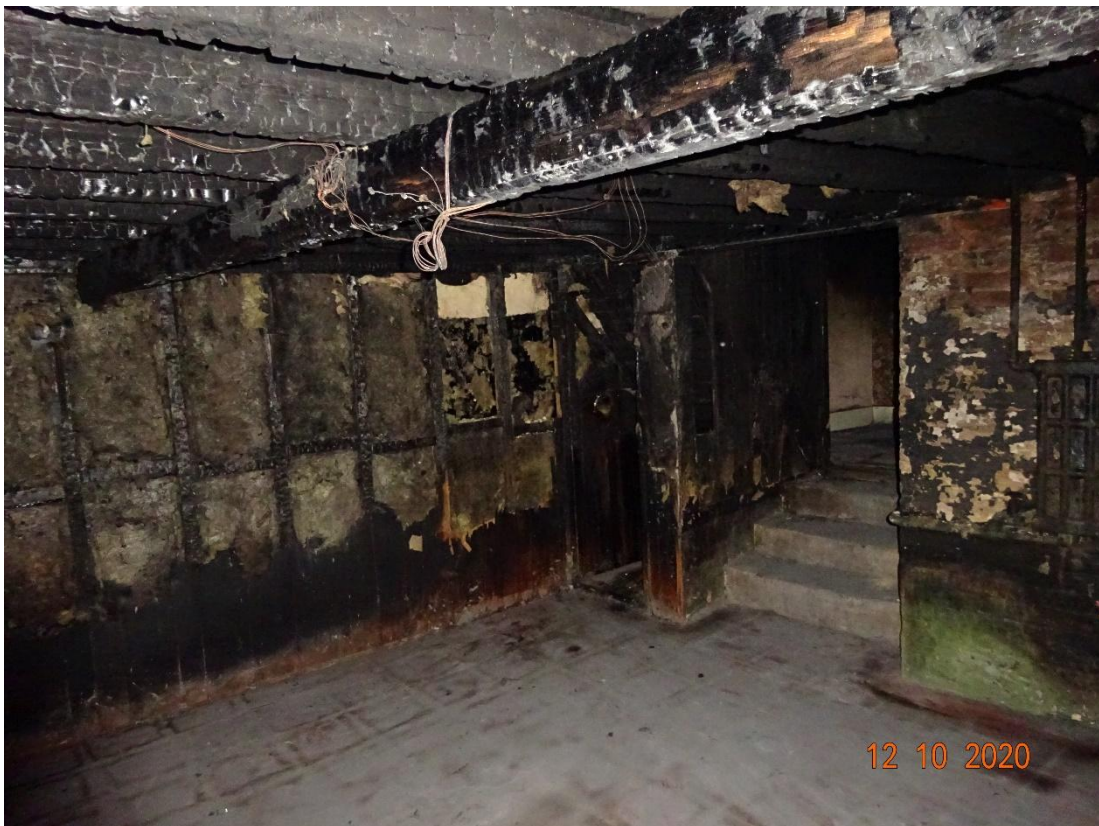
View of fire damaged floor joists in the basement
