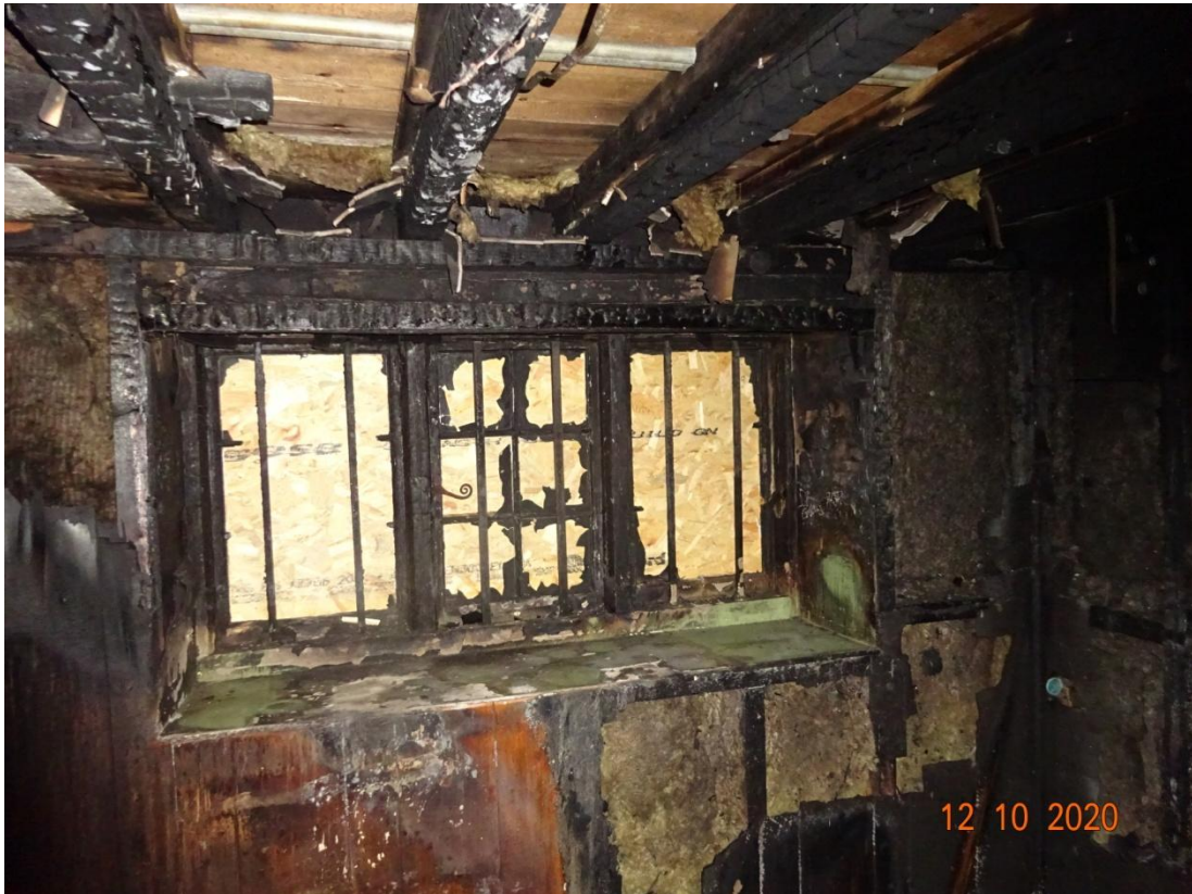
View of fire damaged window in the basement
