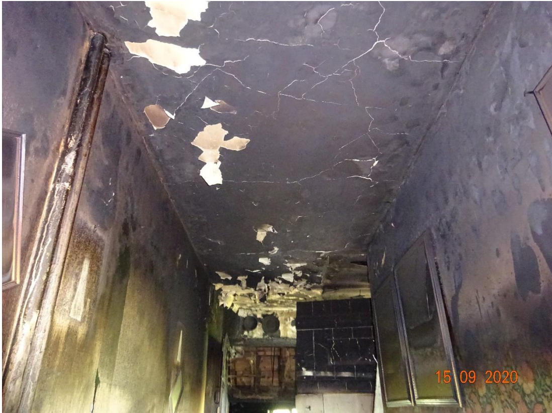
View of fire damaged ceiling in the corridor on the ground floor
