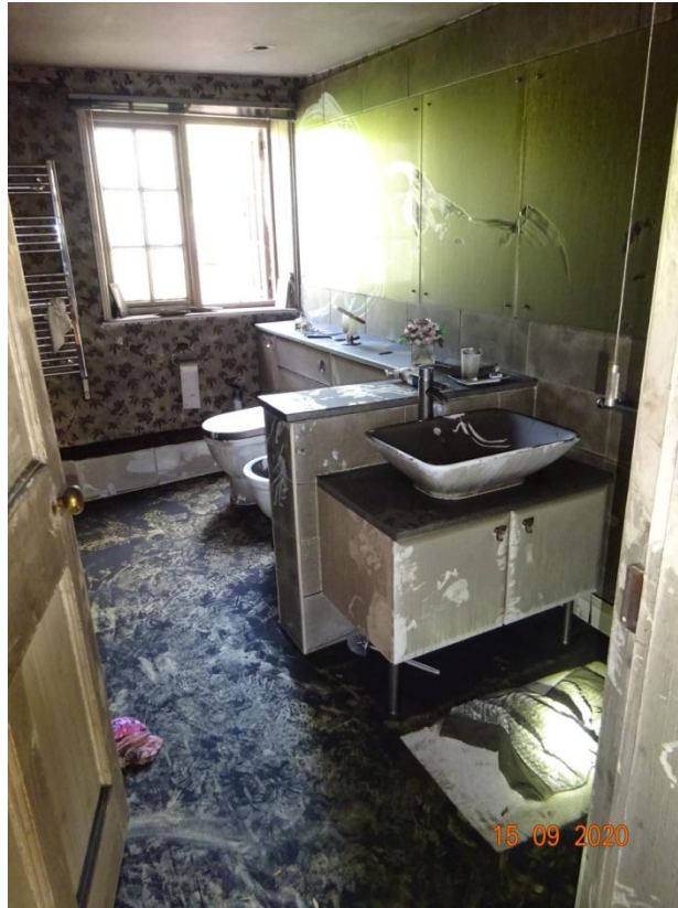
Family bathroom on the first floor after fire
