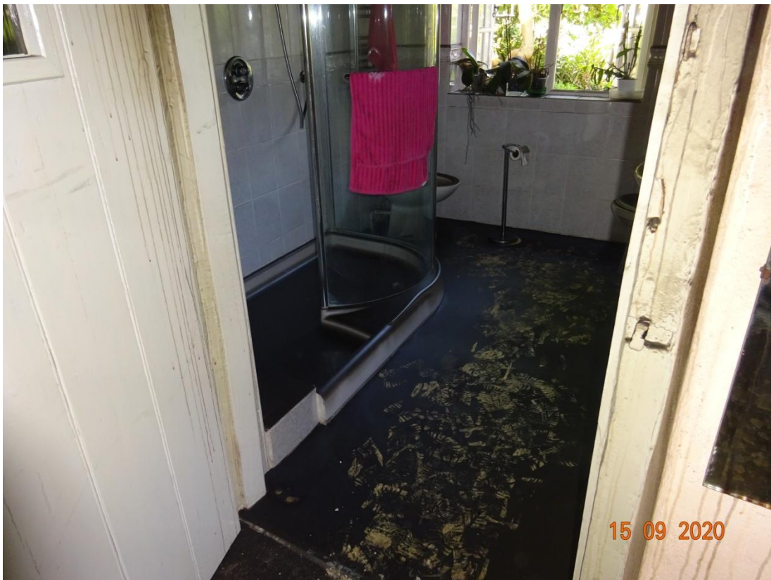
Bathroom on the ground floor after fire
