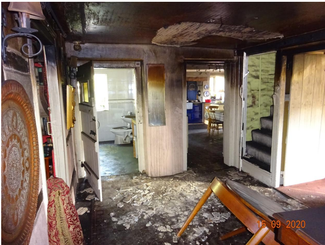
Hall on the ground floor after fire
