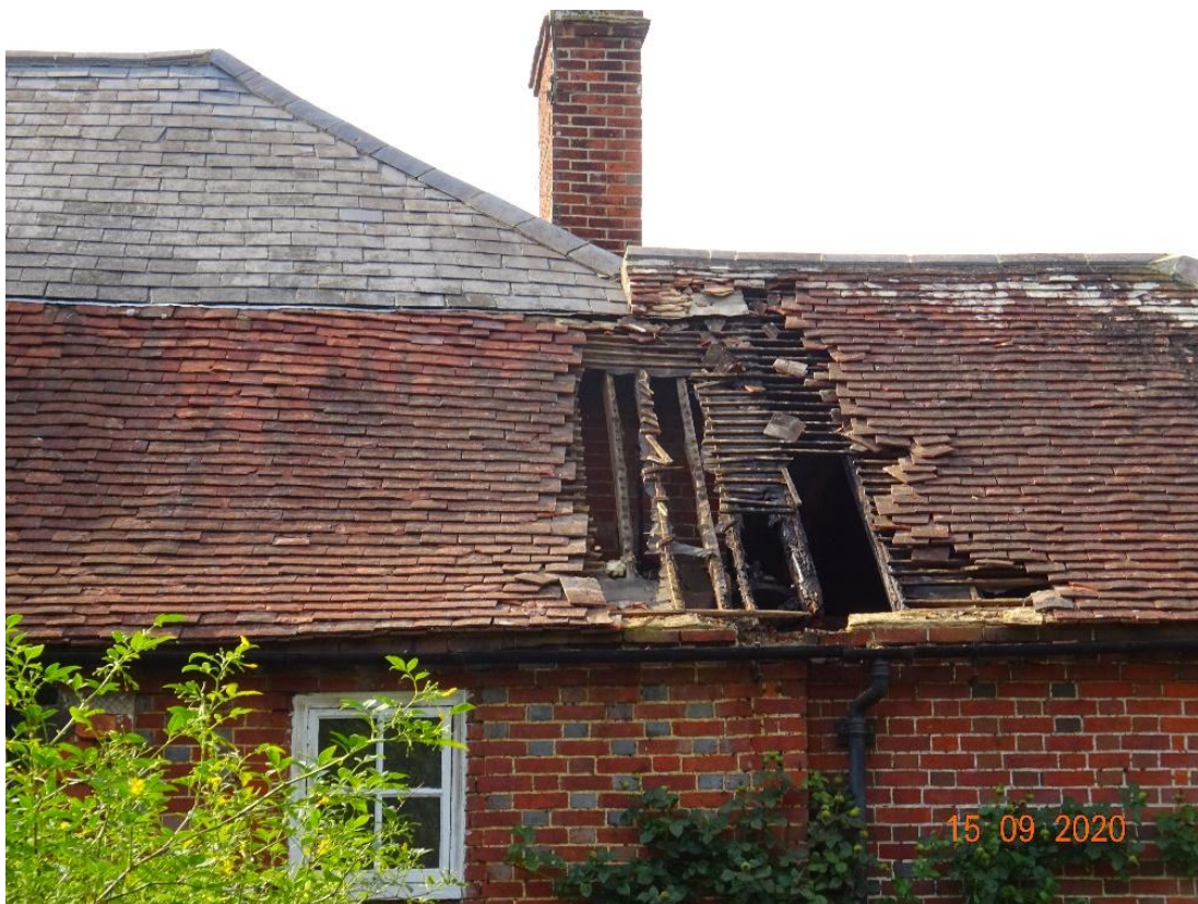
View of damaged part of the roof externally
