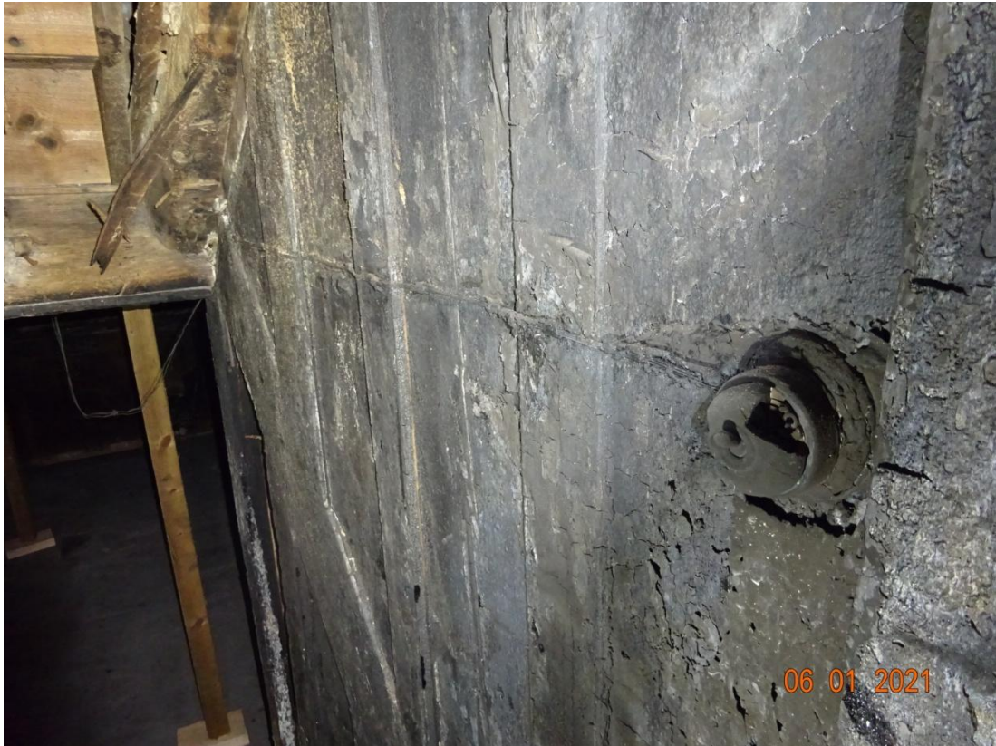
Detail of cladding of the wall between the stairs to the basement
