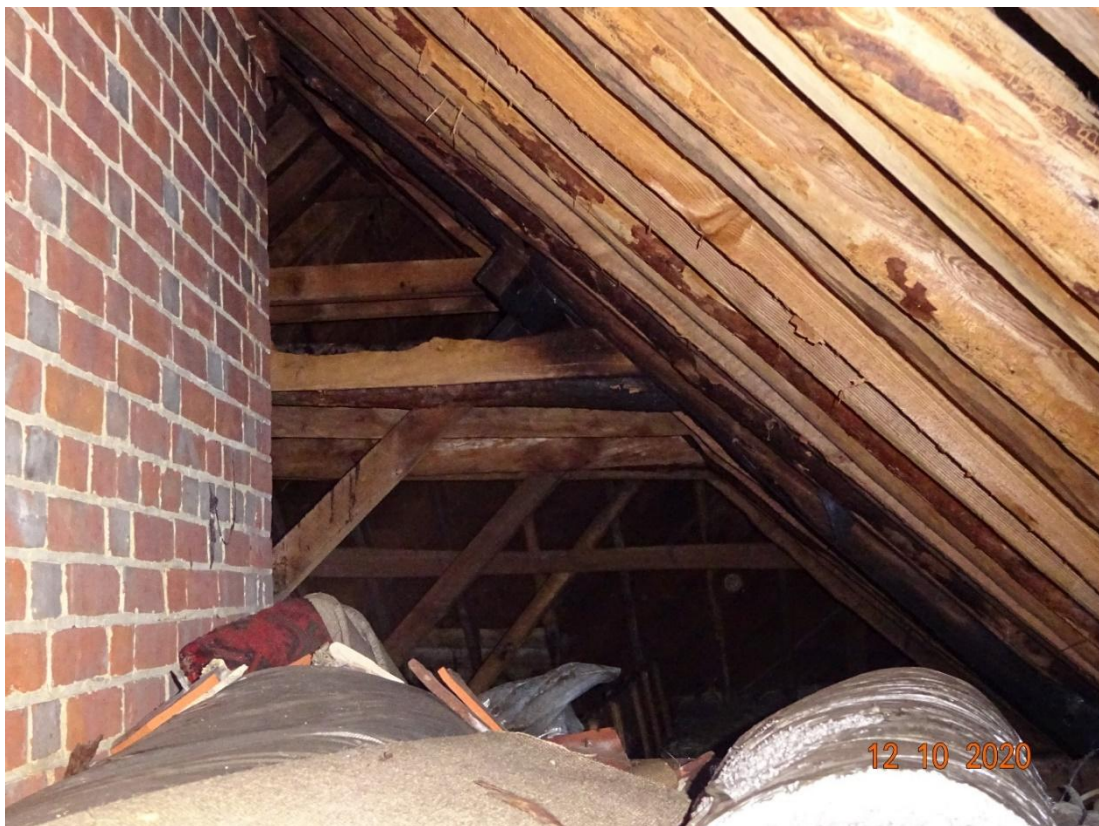
View of damaged part of the roof internally
