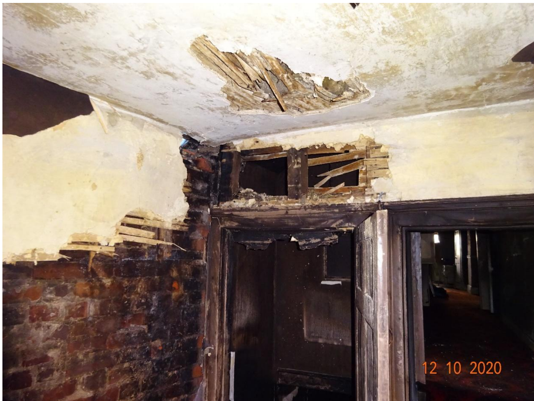
View of fire damaged structure in bedroom 5
