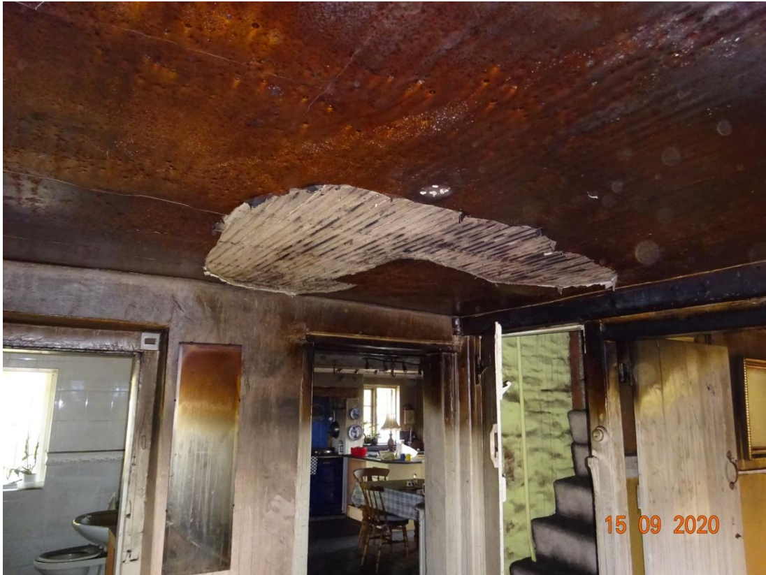
Damaged lath & plaster ceiling in the hall on the ground floor
