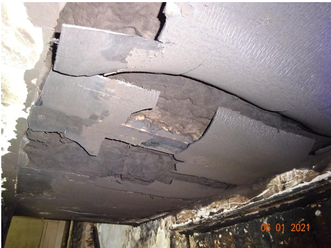
Detail of fire damaged ceiling in the corridor on the ground floor
