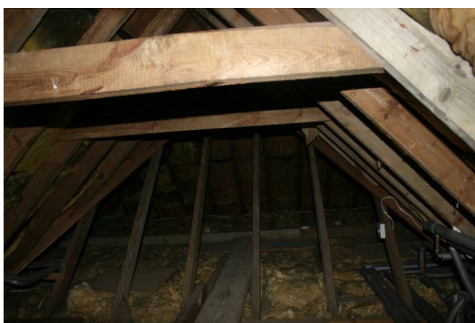
Photo 6: Section of roof over current kitchen, connecting extension roof with original house.
