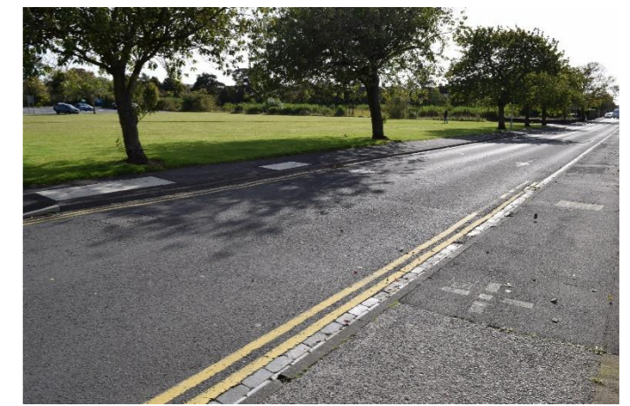
Figure 4.6 Detail of services in Kenilworth Road to the west of Library Gardens and associated slightly raised area within the Site, looking south-east. (Source AECOM Heritage Statement)
