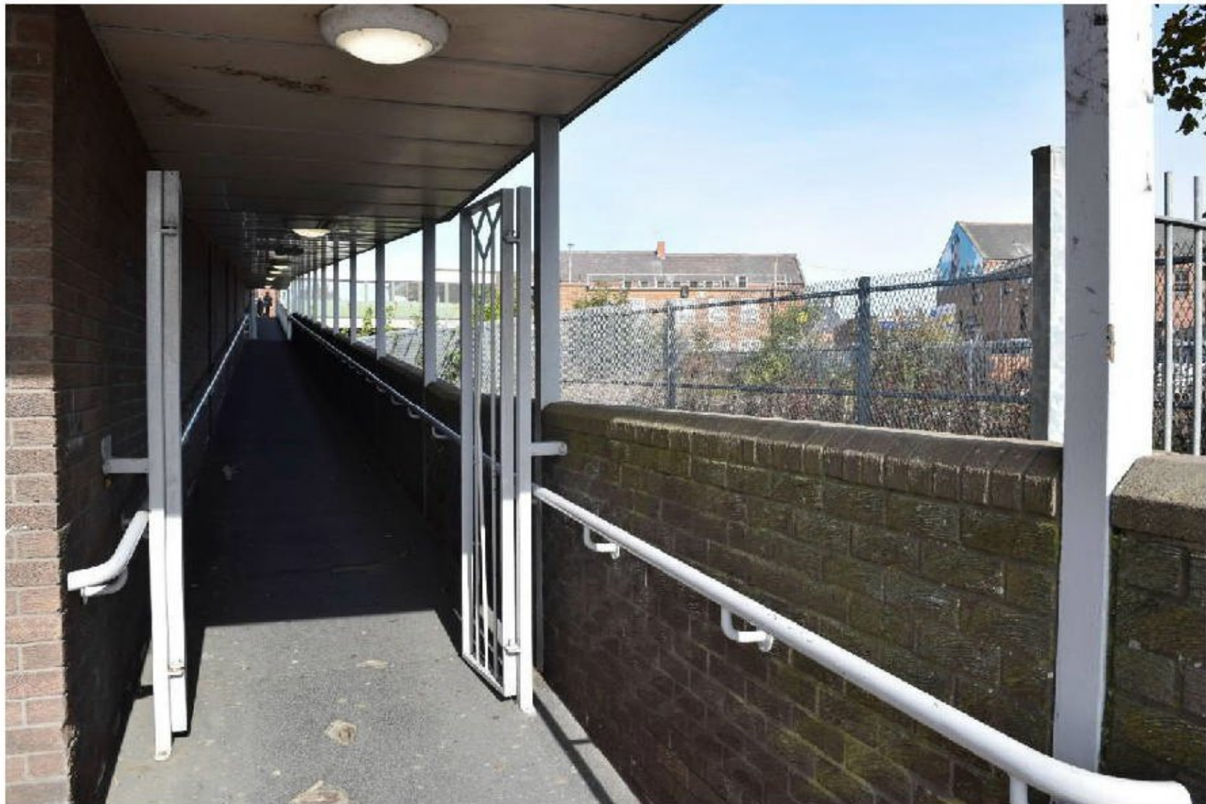
Plate 9. View along the access ramp to the east side of the Wilko building linking the Site to Station Road.
