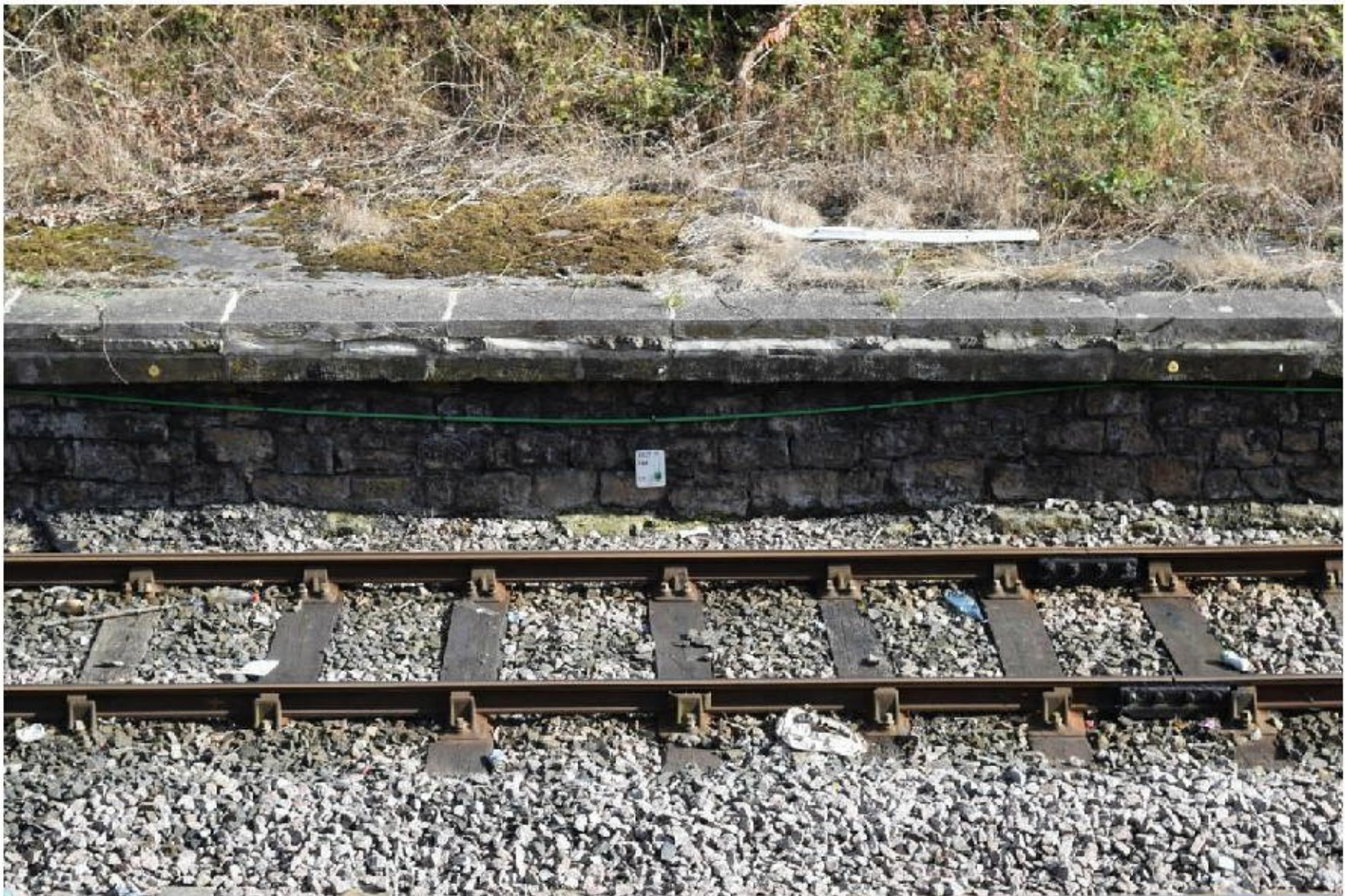
Plate 11. Detail of the stone-built redundant platforms of the former Ashington Station [HNER 27333].
