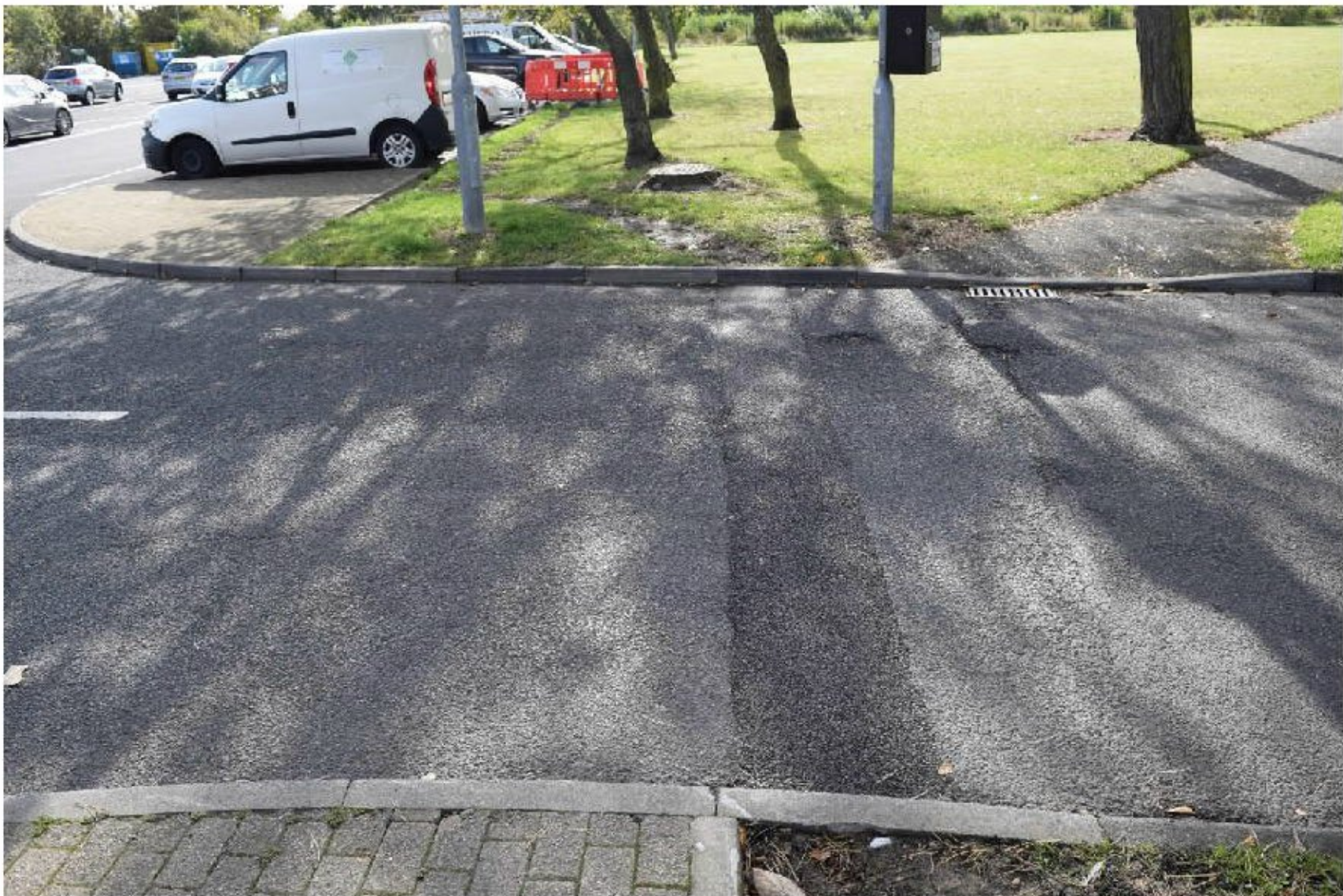
Plate 6. View of the trench for the installation of electric vehicle charging points on the west side of the carpark, looking south.
