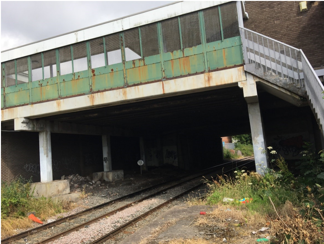
Plate 6. Footbridge connecting Wansbeck Square and John Street Car Park, looking west from former Ashington Station Up platform.
