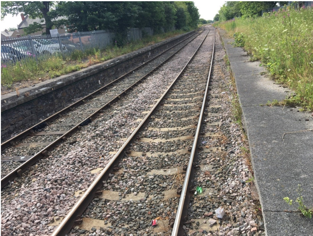
Plate 2. Northumberland Line looking south east from south of the existing footbridge. Former station platforms adjacent to the Up and Down tracks.
