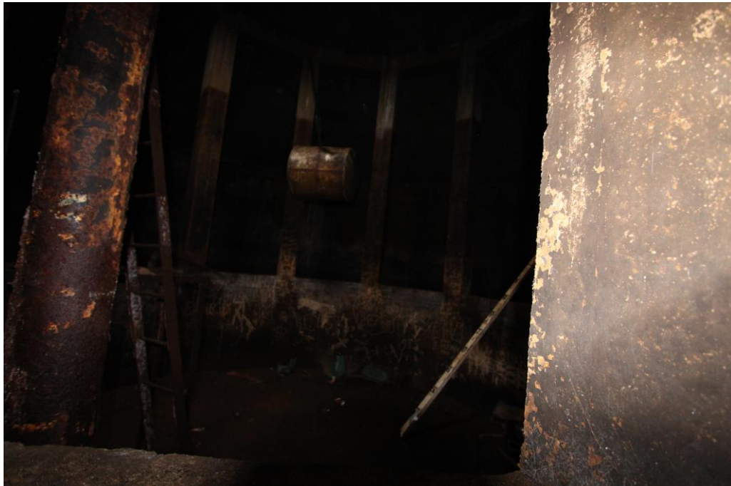
Condition of the cover to the column.
