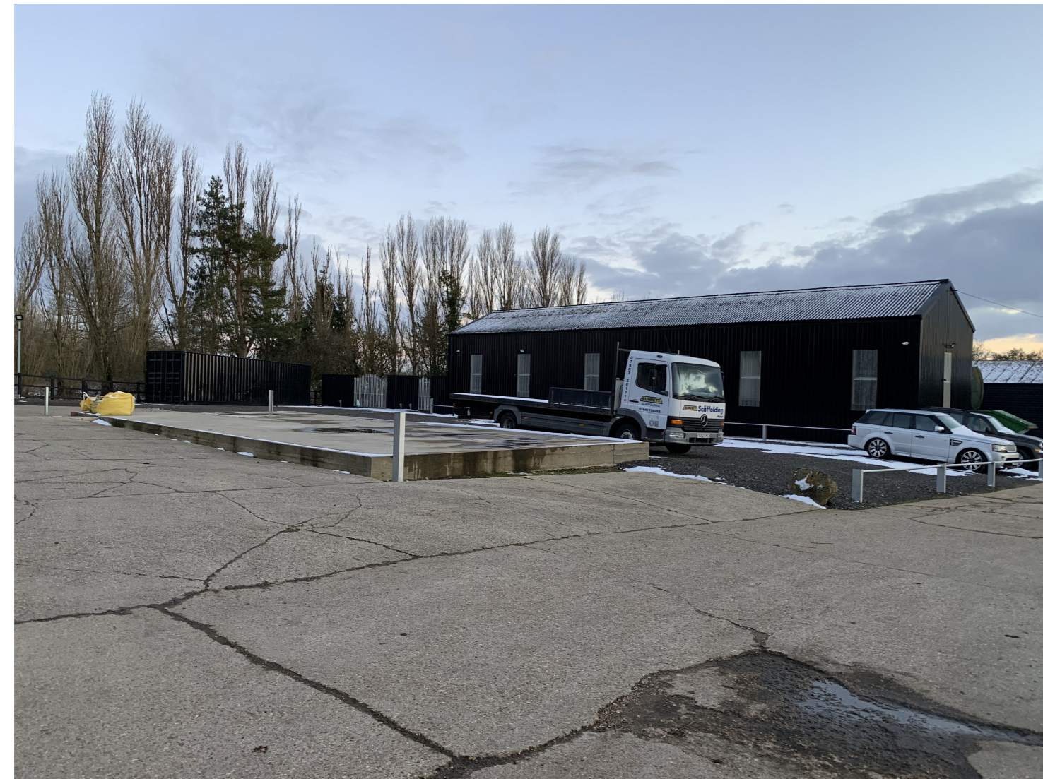
View looking south east towards Building 'P', showing hardstanding area and concrete slab on which new building is to be constructed.
