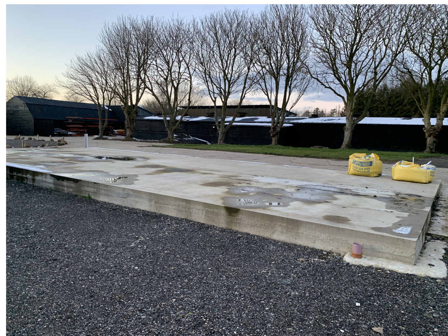
View looking north west towards Buildings 'O' & 'N', showing hardstanding area and concrete slab on which new building is to be constructed.
