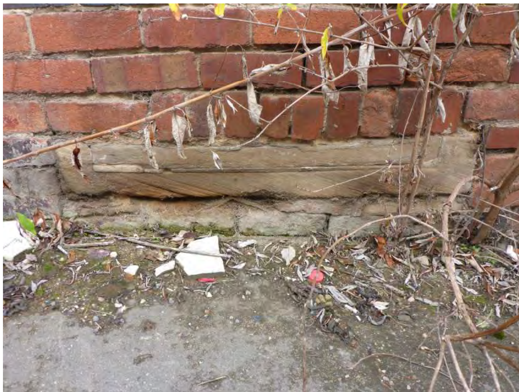
Plate 7: In situ 19 th -century step in fabric of mid-20 th -century building
