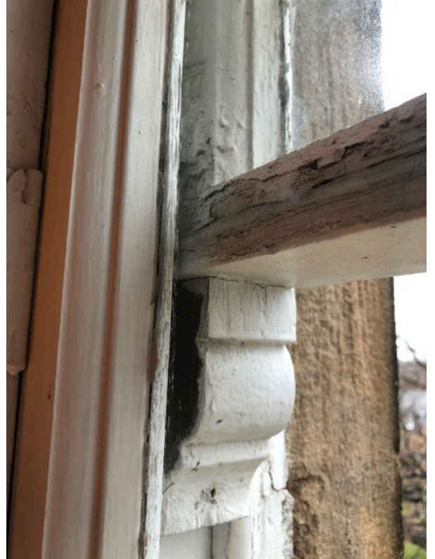
Mid rail rotting and upper style
