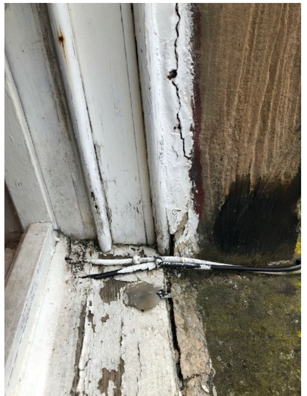
Mastic breaking away
