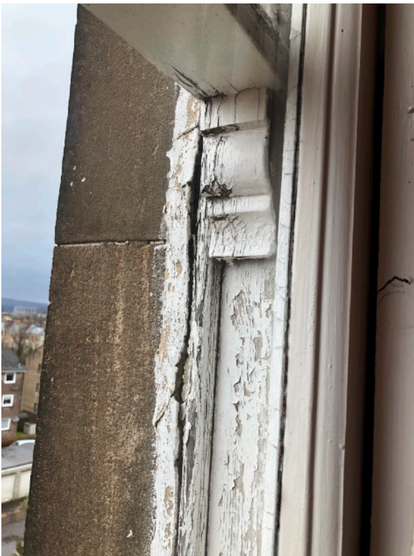
Mastic broken away
