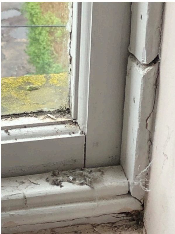
The joint in the newer windows are breaking apart also.
