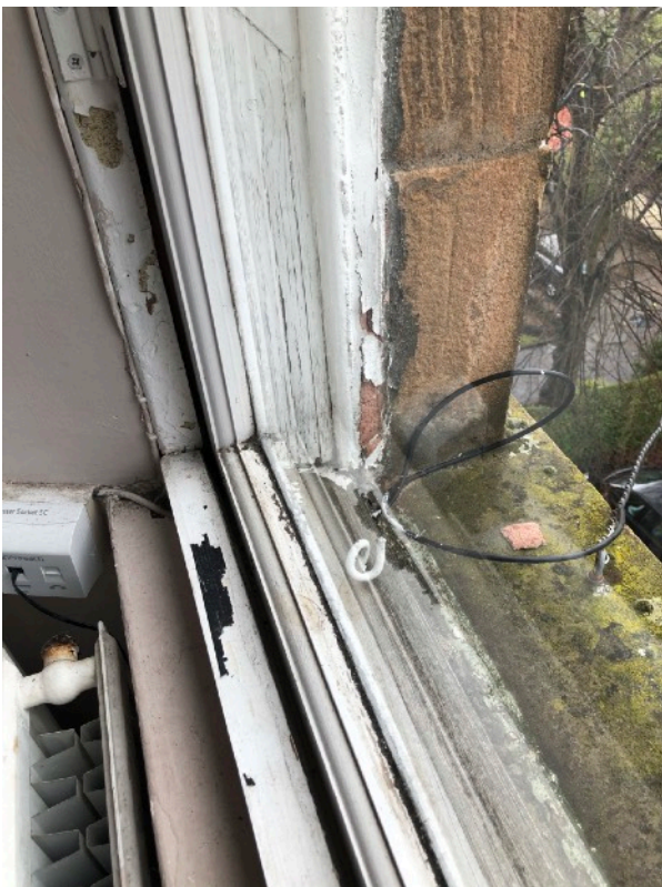
Timbers around windows are rotting
