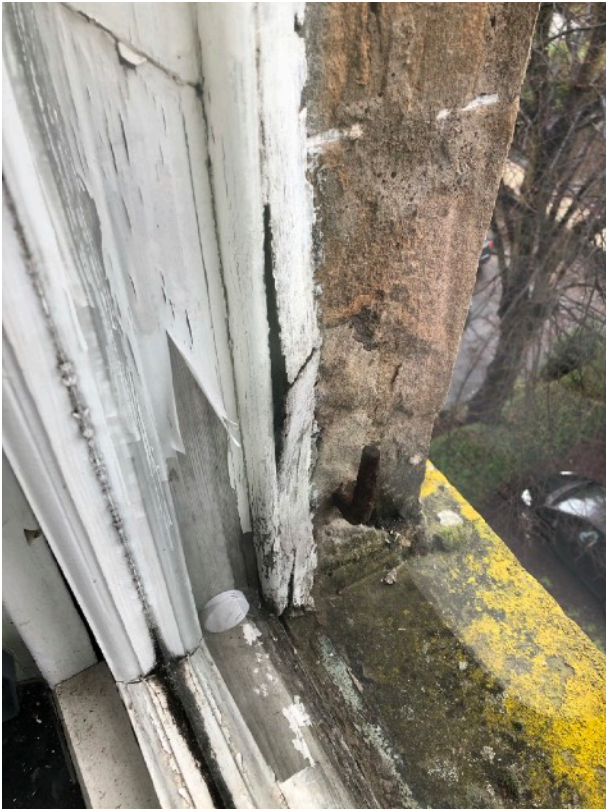
Mould, broken mastic and worn exposed timbers
