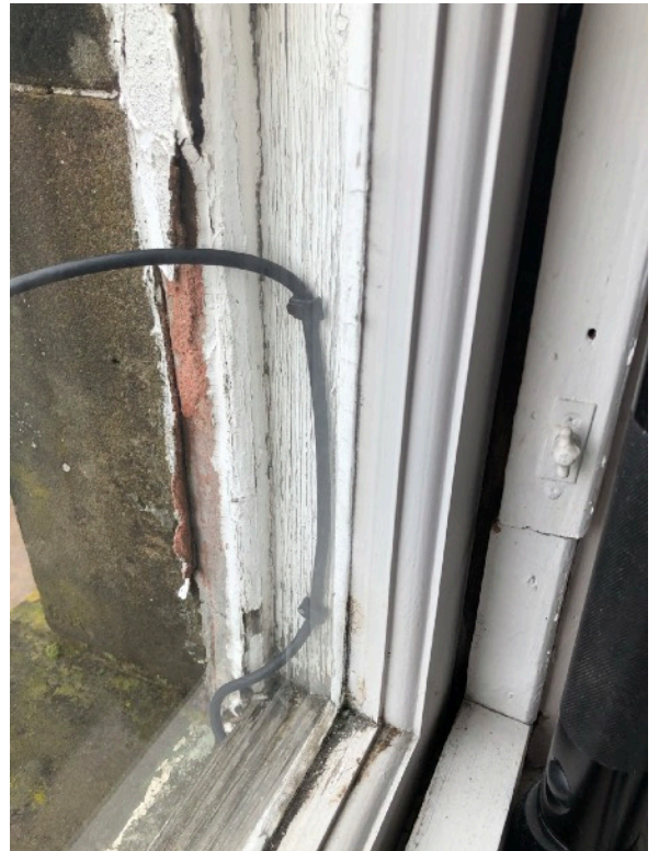
This is a replacement bottom sash but it has not been fitted well, there is also broken stonework that needs repaired
