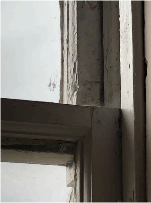
Top sash is original but needs replaced bottom sash is not original but is poorly made and needs replaced
