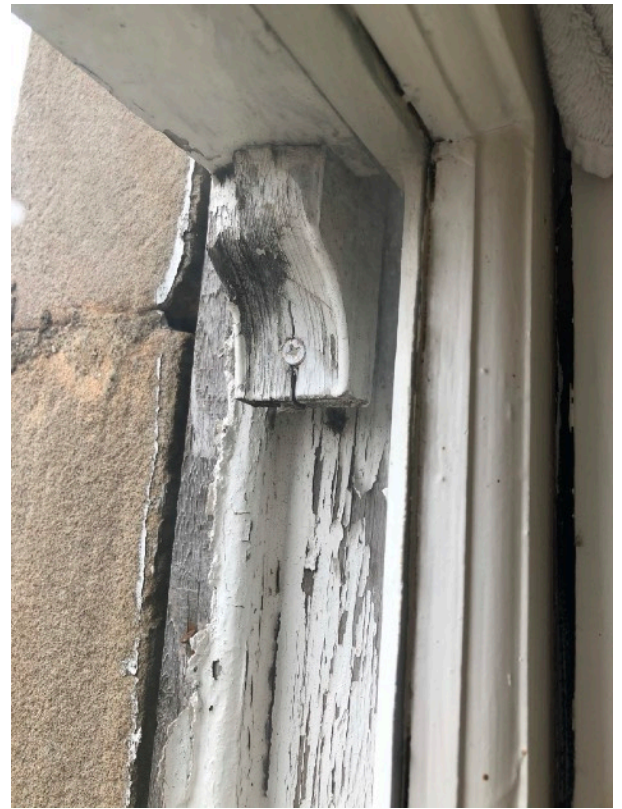
This is the replacements possibly from 1970s that are poorly done and need to be replaced
