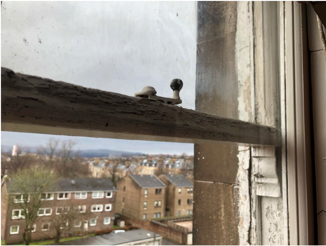
Mid rail rotted
