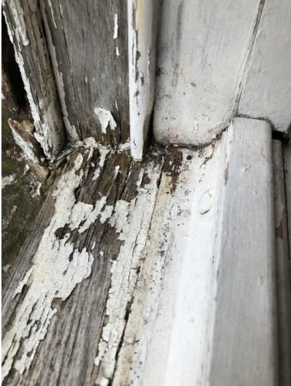
Cill and case breaking and rotting
