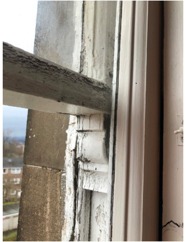
Rotted mid rail
