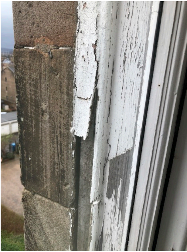
Mastic breaking away, exposed and rotted timbers
