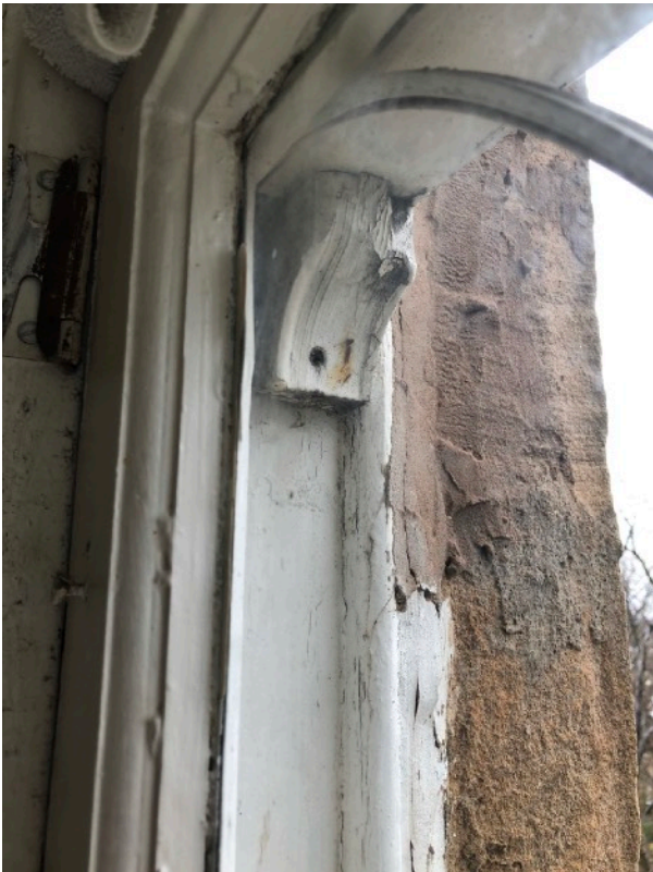
The top sash has been replaced years ago as indicated by the curved horn which is not original, the replacements were not fitted well and leave draughts
