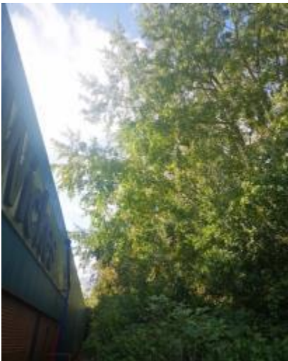
Figure 4: G1 overhanging building.
