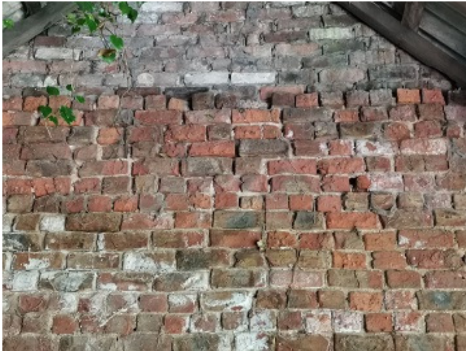
Plate 8. Example of holes in internal wall of Building 3
