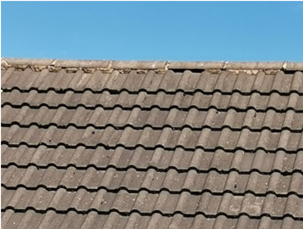
Plate 14. Shows gaps under ridge tiles on Building 6
