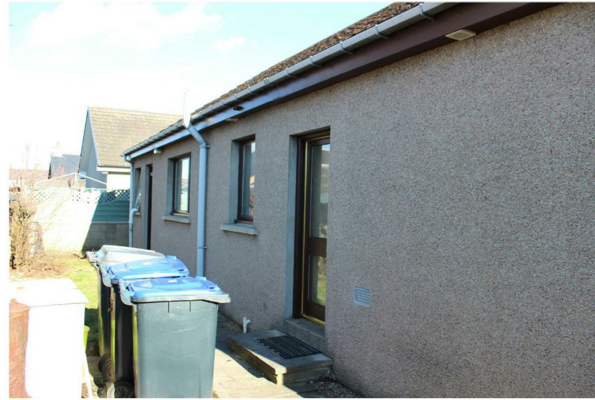
WEST ELEVATION FROM GARDEN: Garage Window No.1 & Door, Bedroom Window, Bathroom Window & Kitchen Rear Entrance Door.
