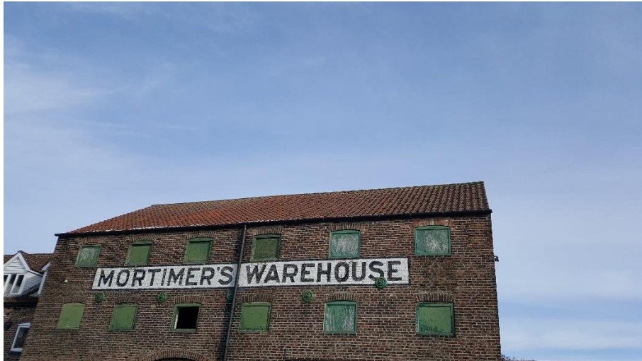
Plate 8: the pitched tiled roof of the warehouse. Photograph taken from the west.
