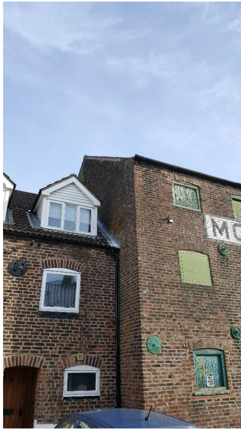
Plate 1: the connection between the warehouse and the neighbouring residential property. Photograph taken from the west.
