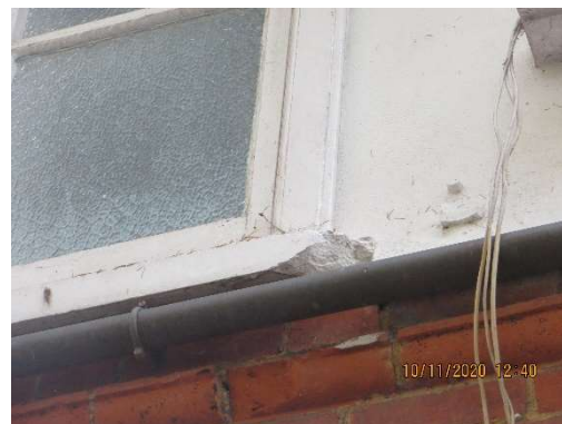
Photo 4 – damaged concrete sill
