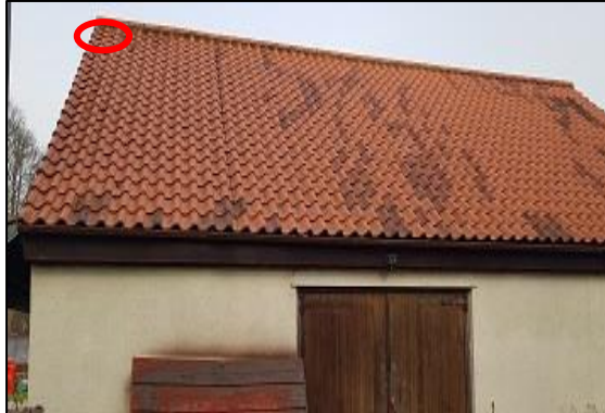
Figure 3: Location of lifted tile circled red.
