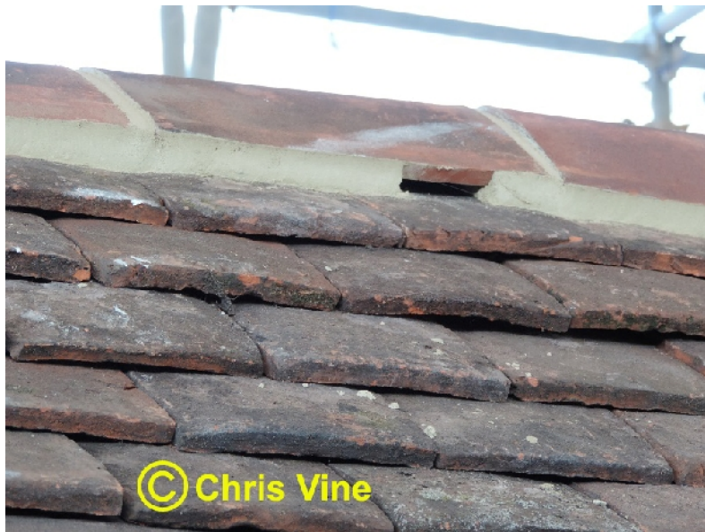
Photo 1. Example of bat access point under newly fitted ridge tile.
