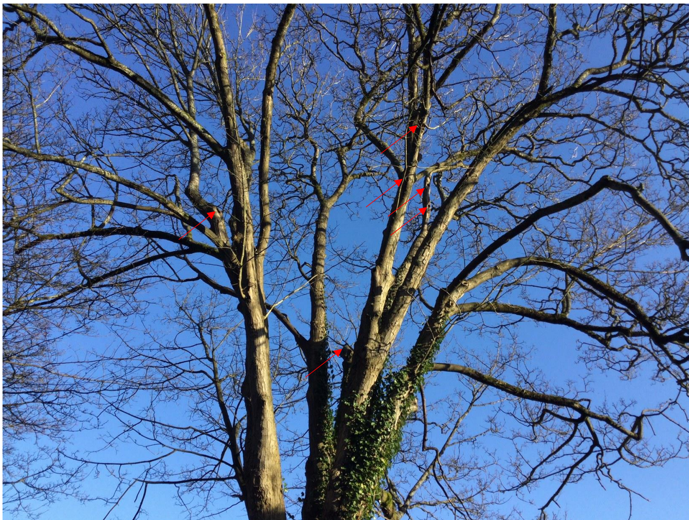
SAL1 T2 sycamore with woodpecker holes, decay and failed branches evident (shown by red arrows).
