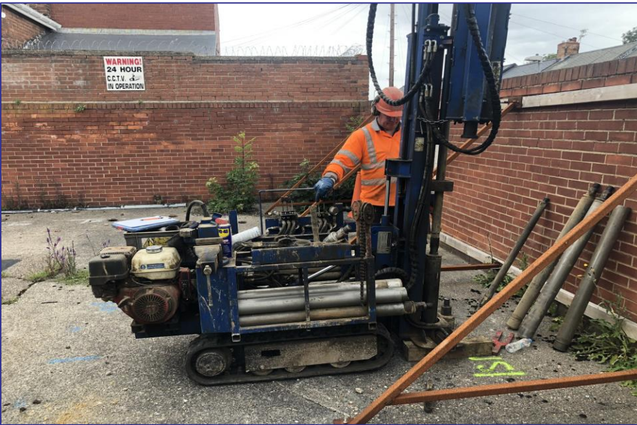
Photographic Plate 3 – Window sampler drilling rig advancing borehole WS1 next to tank farm.
