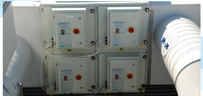
4 ESP Units Stacked in modular formation with a double pass
