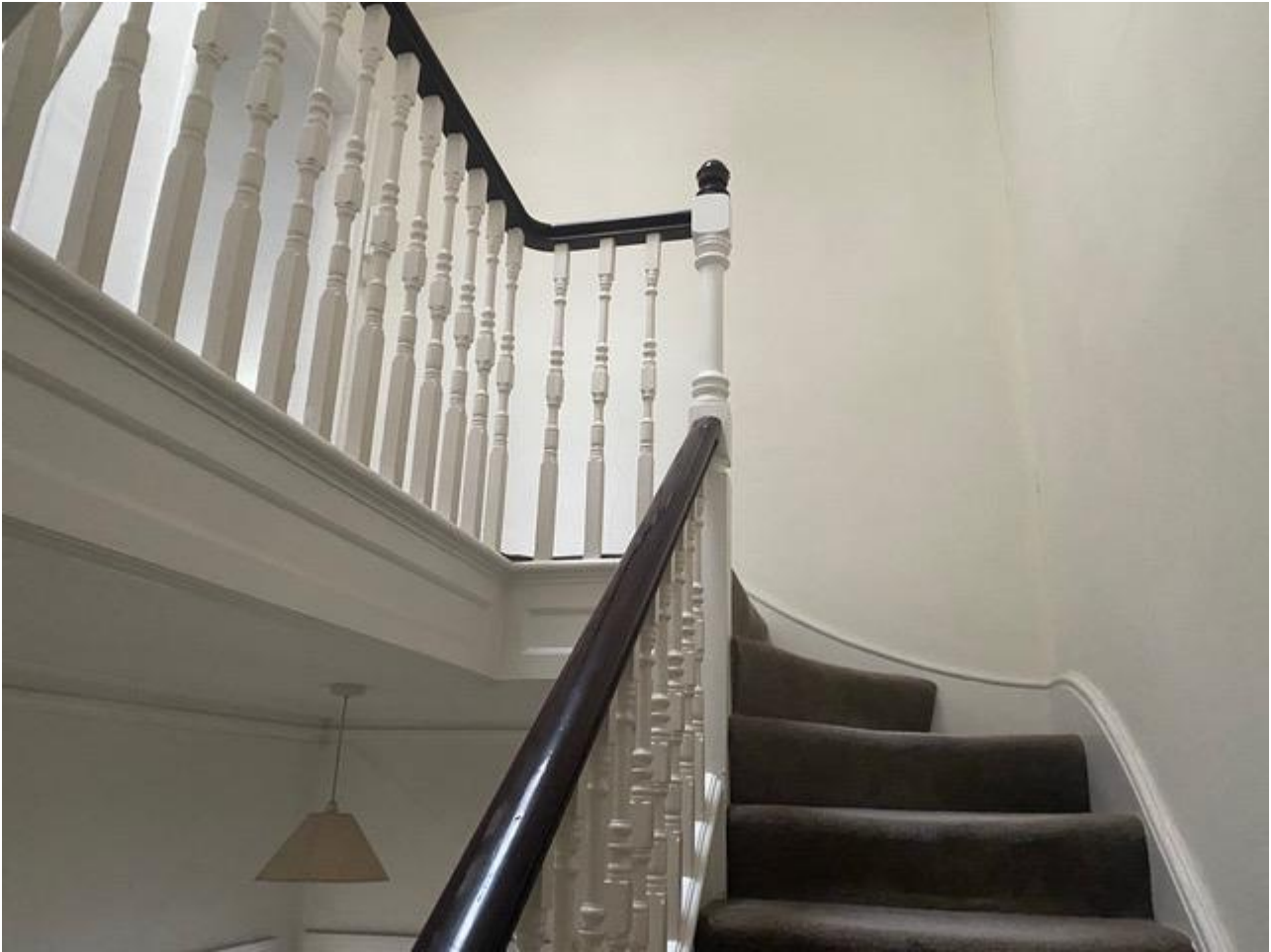
Figure 10 - The upper staircase, of broadly late Victorian or Edwardian date, between the third and fourth floors in 40 Montagu Square.
