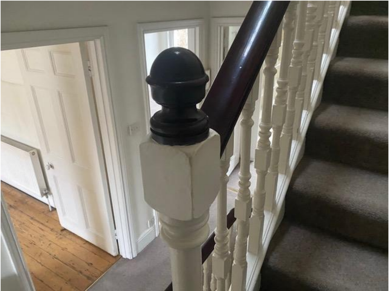
Figure 9 - The upper staircase, of broadly late Victorian or Edwardian date, between the third and fourth floors in 40 Montagu Square.
