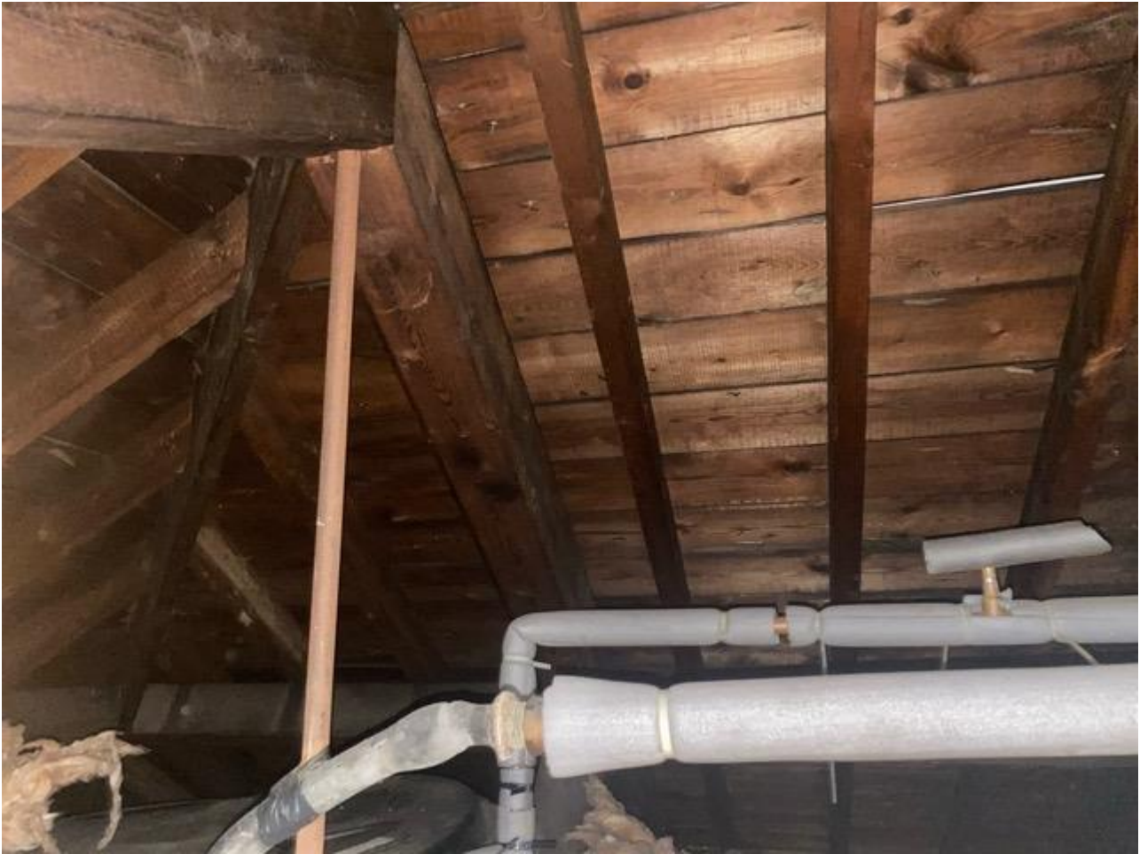
Figure 6 - The interior of the hipped roof, of late 19 th or early 20 th century date.
