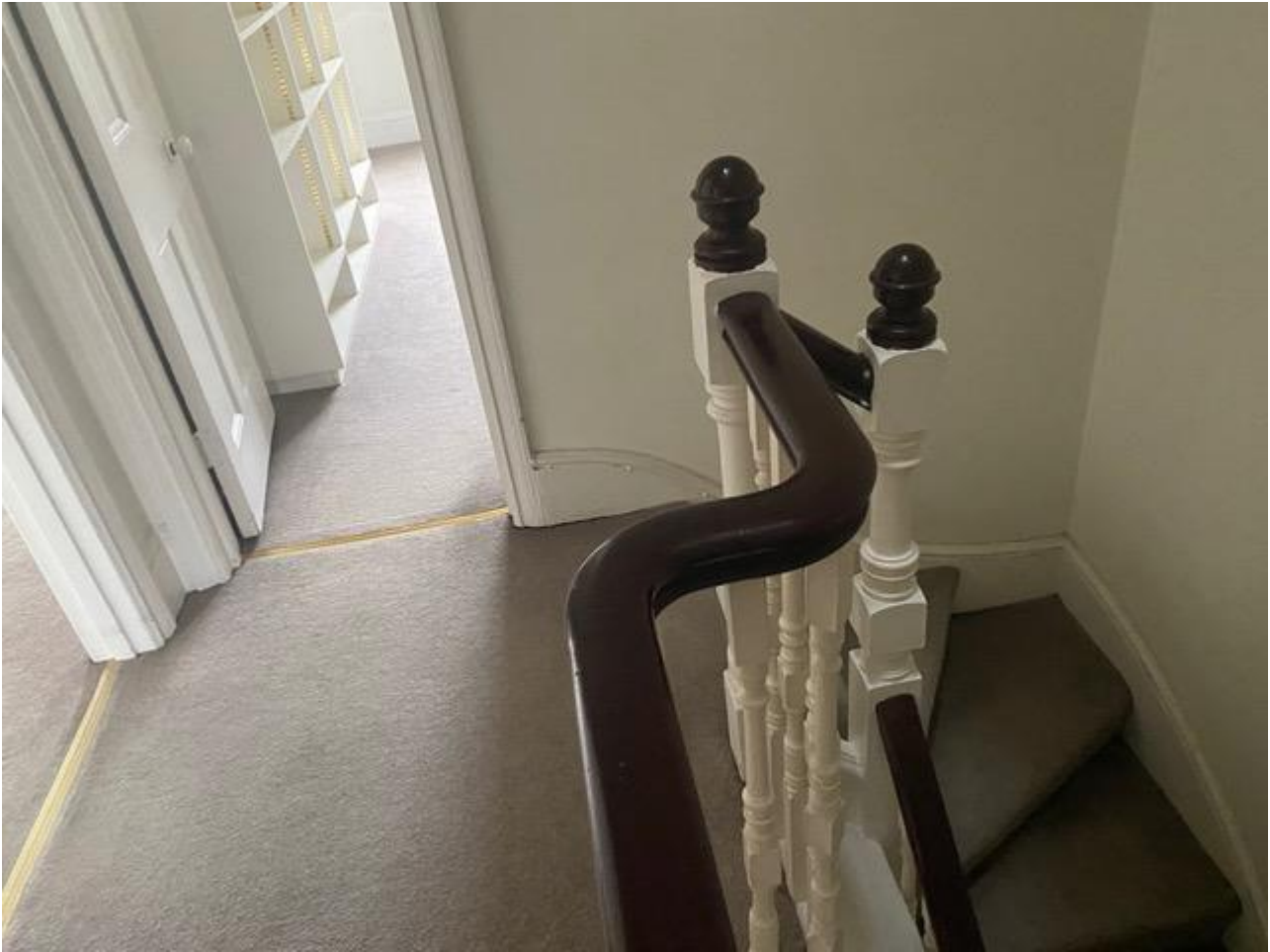
Figure 11 - The landing of the upper staircase, of broadly late Victorian or Edwardian date, third floor, in 40 Montagu Square.
