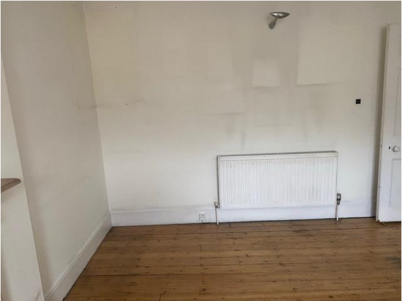
Figure 15 - Dividing wall between the third floor front and back rooms, seen from the back room (kitchen) looking towards the front.
