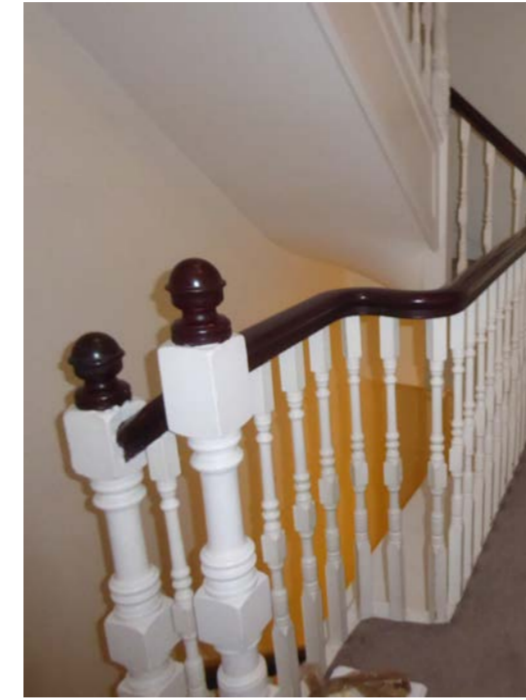
Image 4_ The 3rd floor landing; The stair balustrade and handrail are proposed to be reconfigured to remove the kink in the hand rail and increase the width of the landing.
