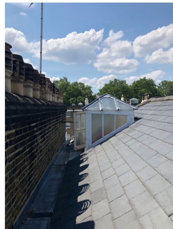
Image 2 _The existing single-glazed roof lantern as viewed from the east. It provides light to the stairwell below, whilst also serving as a means of access for both the roof and the loft.
