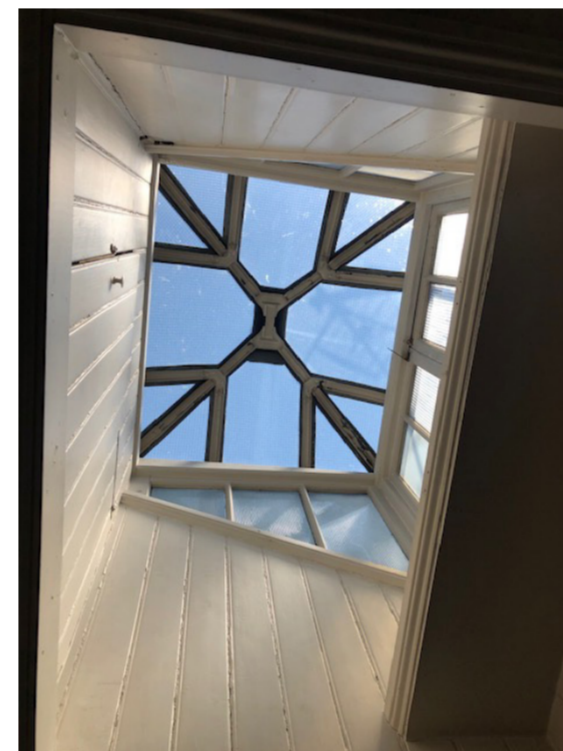
Image 4 _The roof lantern as viewed from the landing, including the small shelf (to the right of the image) that currently provides access to roof, in tandem with a freestanding ladder, that is stored on the landing.
