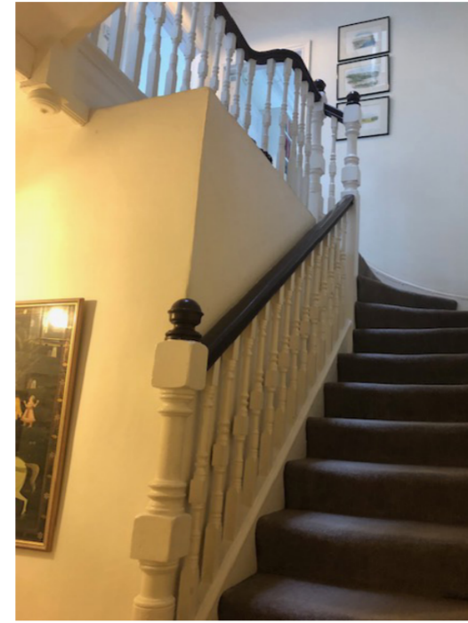
Image 3_ Stairway to the 3rd floor; The stair balustrade and handrail are proposed to be retained and refurbished generally.
