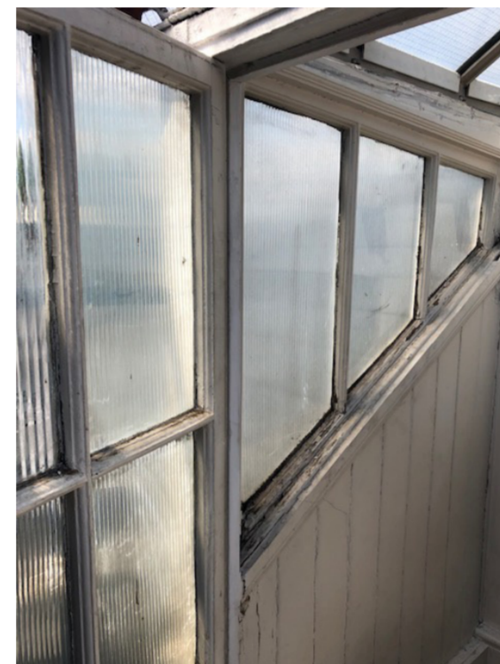
Image 3 _The timber and glass construction of the existing roof lantern. The glazing is single glazed 'reeded' glass. The timber is worn.
