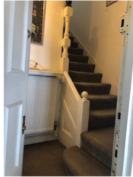
Image 2_ The entrance lobby; The stair balustrade is proposed to be retained and refurbished generally.
