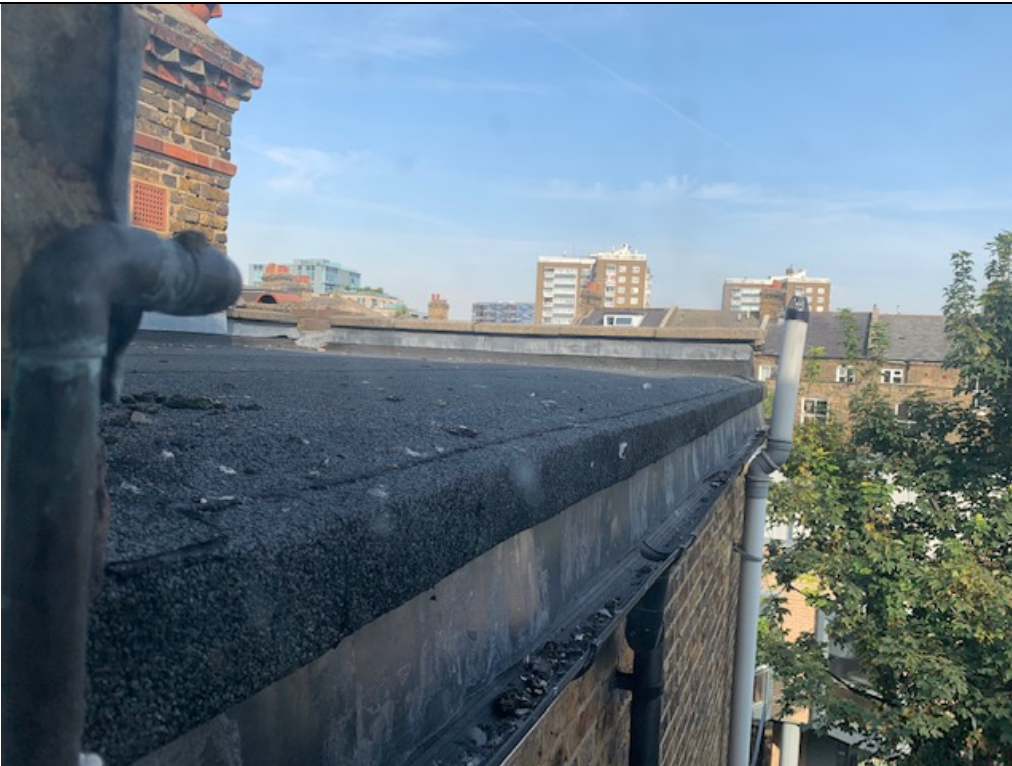
8. Close-up of felt-covered flat roof. To have new liquid coating from Kemper System or similar.
