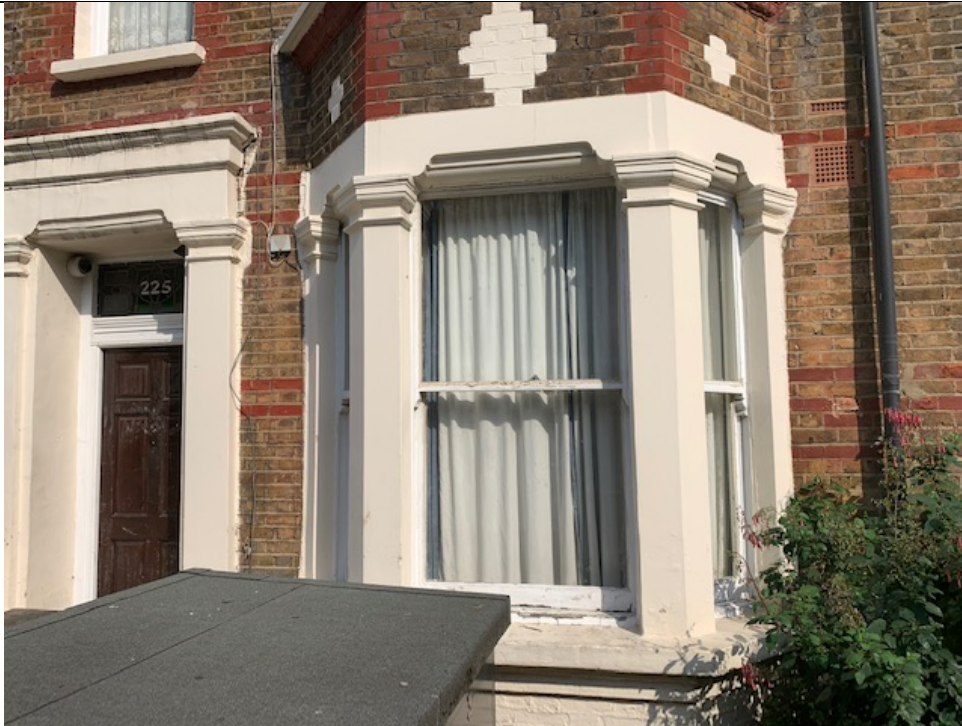
3. Close-up view of ground floor bay window with sashes, and front door.
