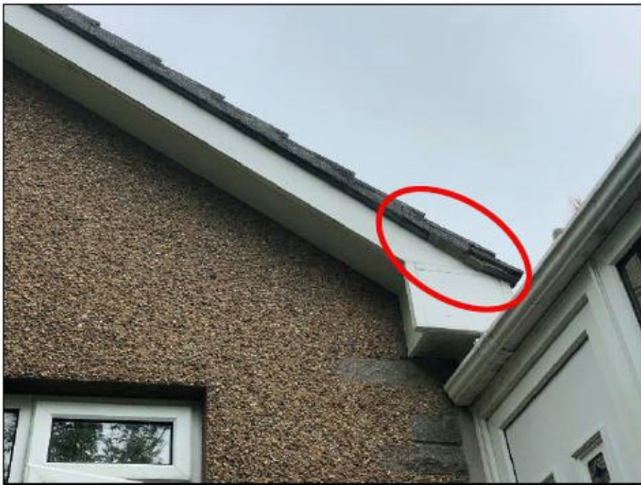
Figure 4 Gaps in roof tiles
