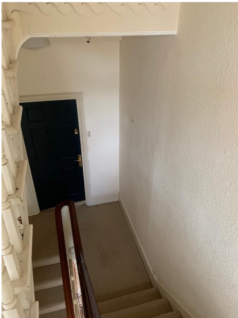
Fig 2 - Front Door of First Floor Flat, 21 Downleaze to be relocated to the wall to its right.
