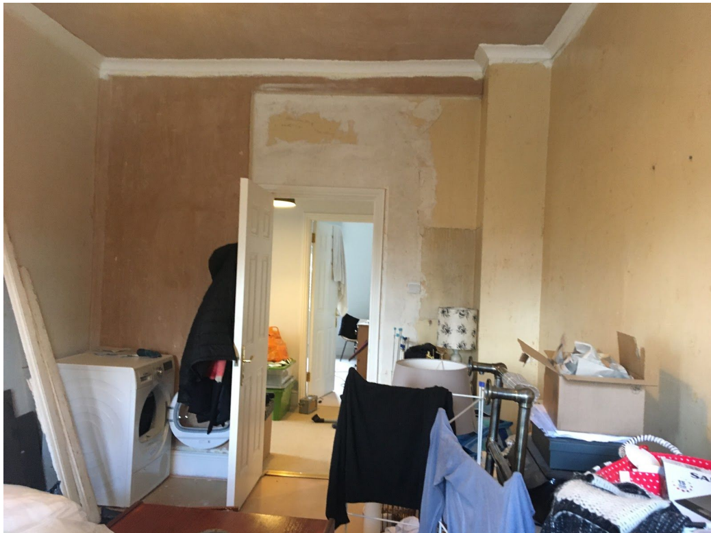
Fig 8 : View of bedroom inside first floor flat. The walls to the left and rear of the photograph and doorway were built in the 1970s. The coving and skirting was also added in the 1970s conversion. It is proposed to build a new stud wall here to form the new entrance lobby.
