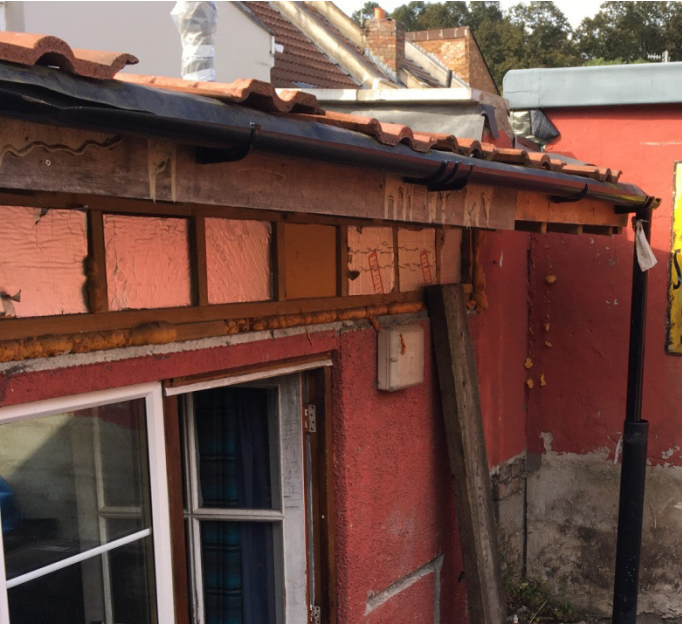
2. Single storey Use Class C3 area with flat roof. Boundary with no.300 North Street with roof line of extension within no.300 visible.
